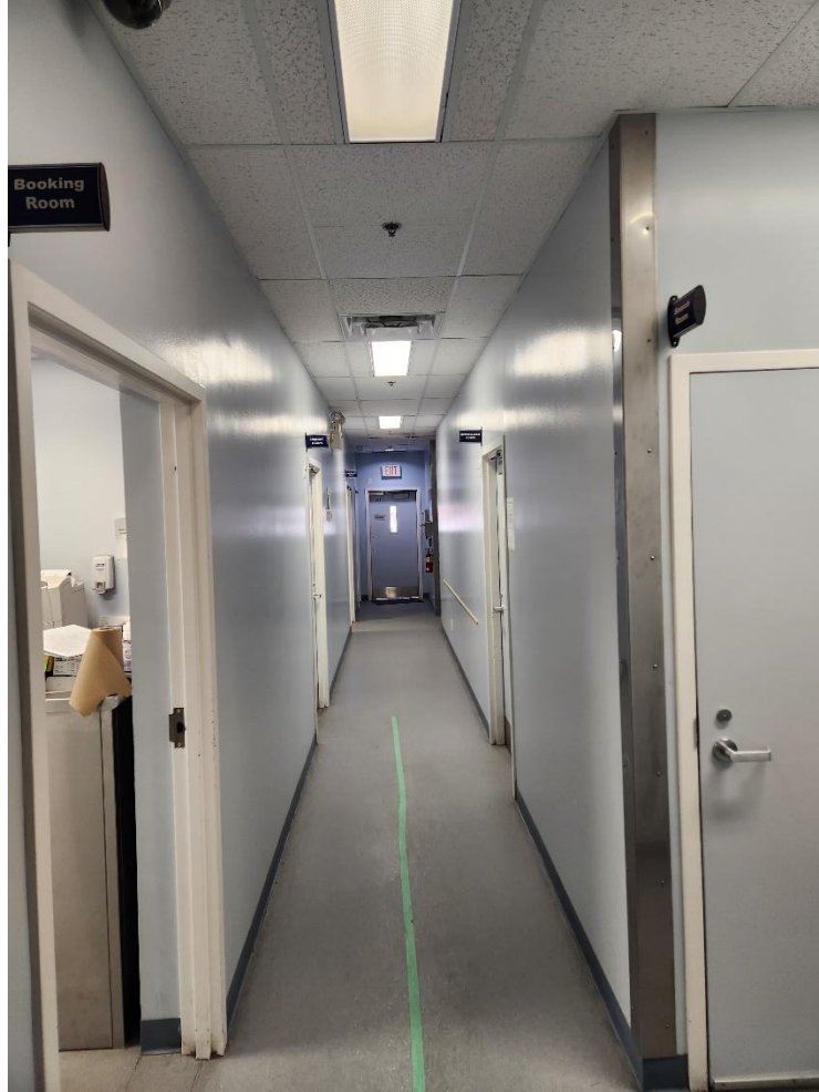
Photograph # 20 1 by 4 Hallway Lights and Red Exit Sign
