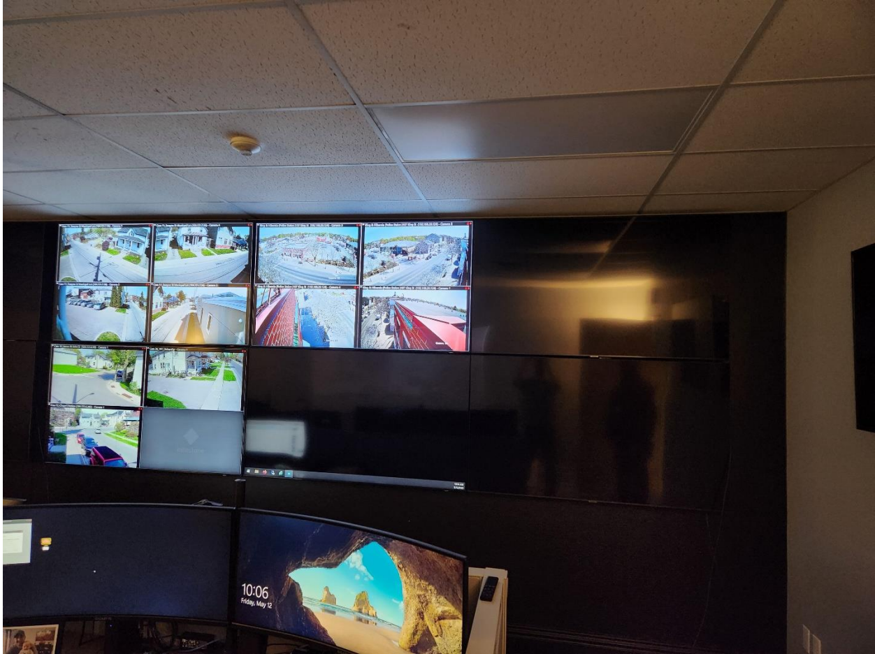
Photograph # 81 Security Surveillance Room
