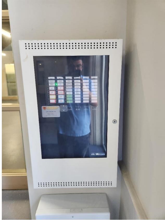
Photograph # 80 Fire Alarm System Panel
