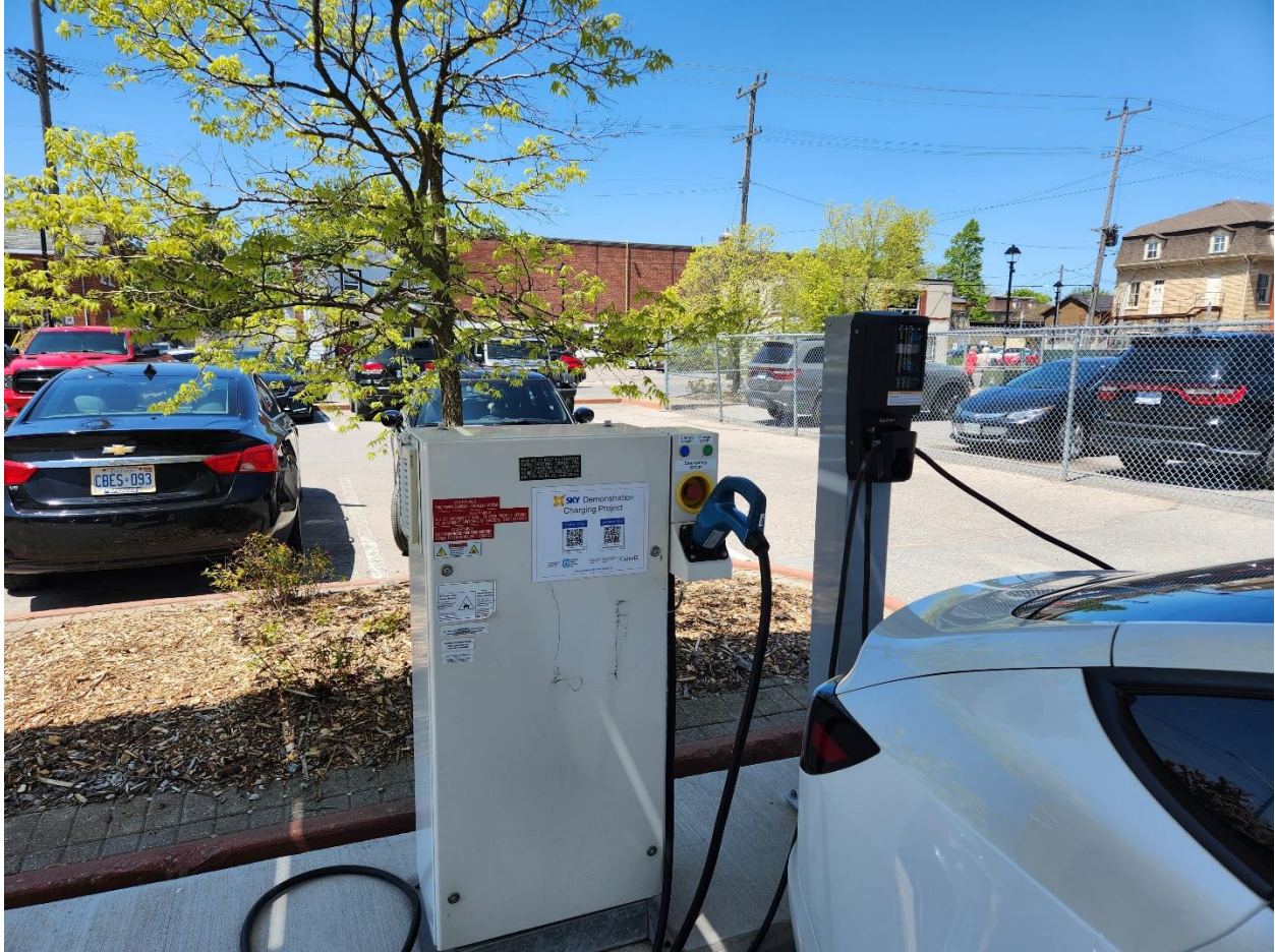
Photograph # 88 6kW DC Fast EV Charger
