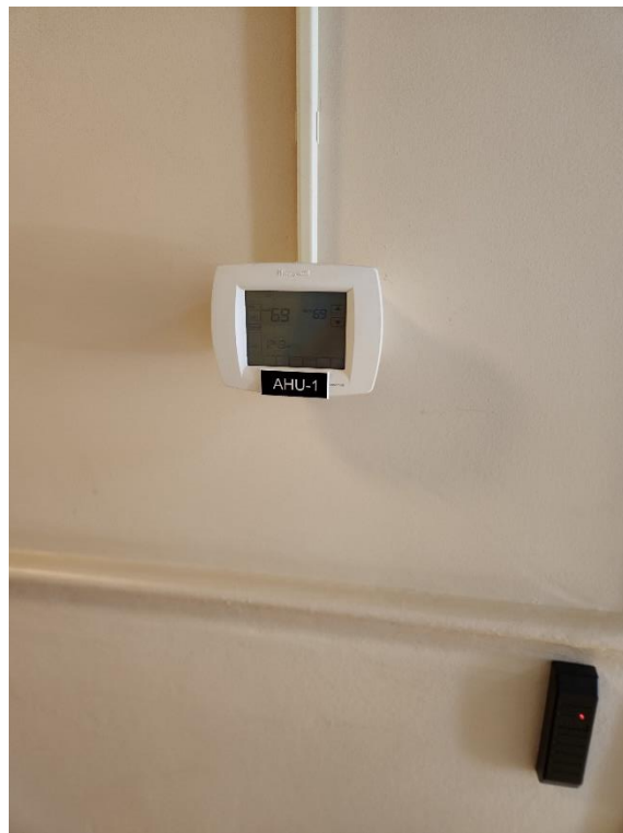
Photograph # 44 Furnace Wall Controller
