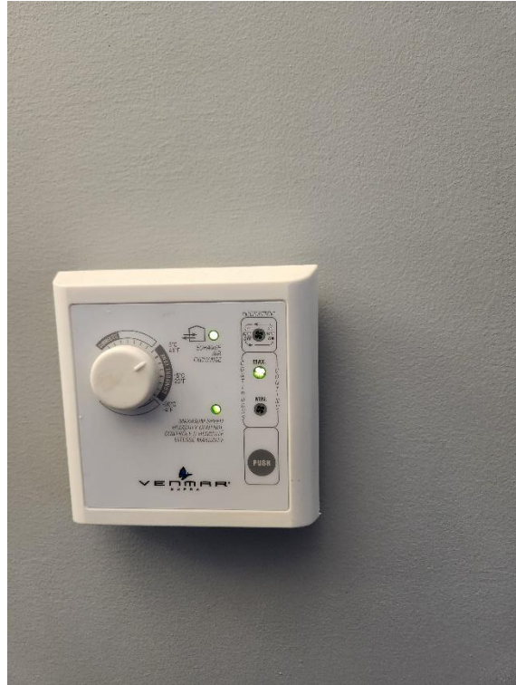
Photograph # 43 ERV Controller
