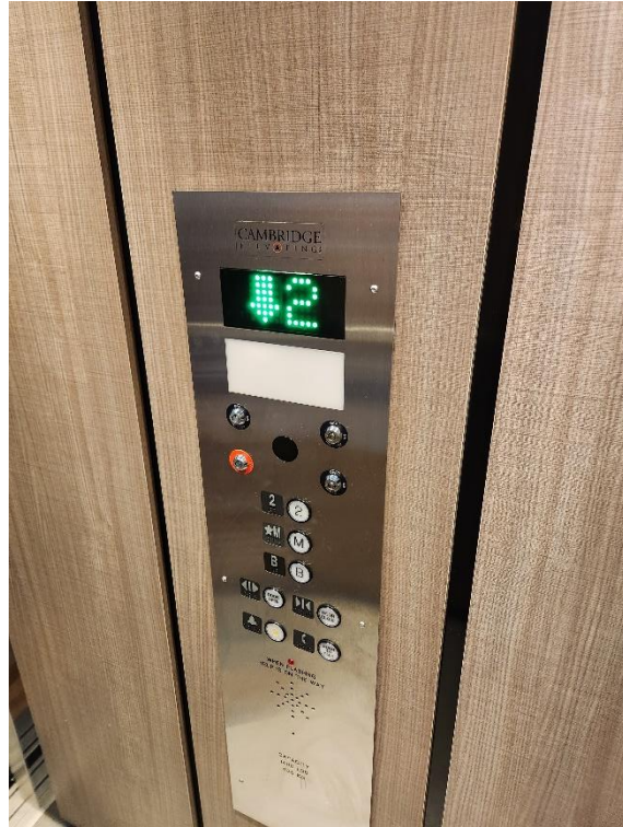
Photograph # 5 Elevator Control Panel
