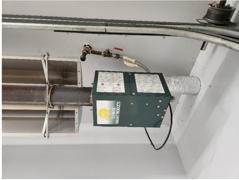
Photograph # 10 Natural Gas Infrared Heater
