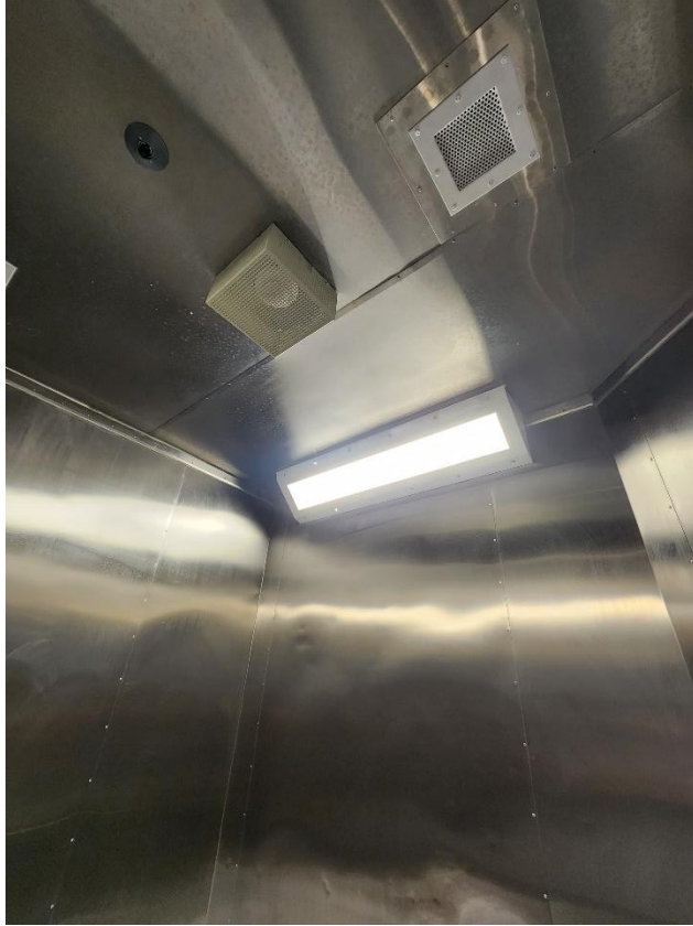
Photograph # 22 1 by 4 Light Fixture with Additional Plexiglass Covering
