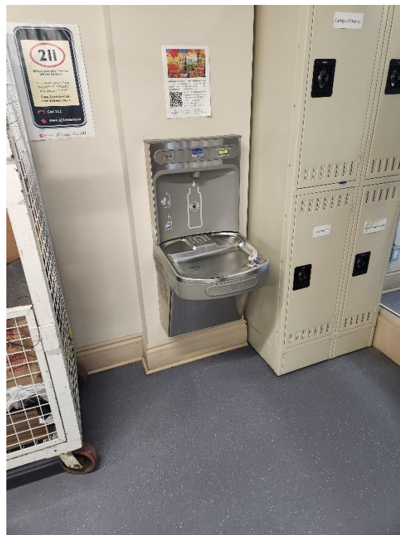
Photograph # 21 Dual Water Bottle Refill Station and Drinking Fountain
