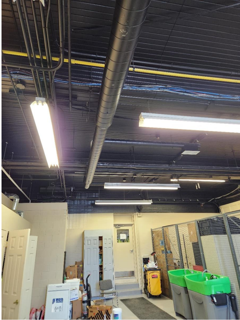
Photograph # 77 T5 Fluorescent Light Fixtures
