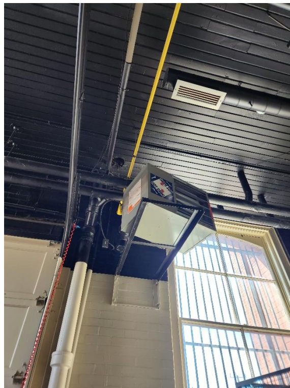
Photograph # 31 Natural Gas Unit Heater
