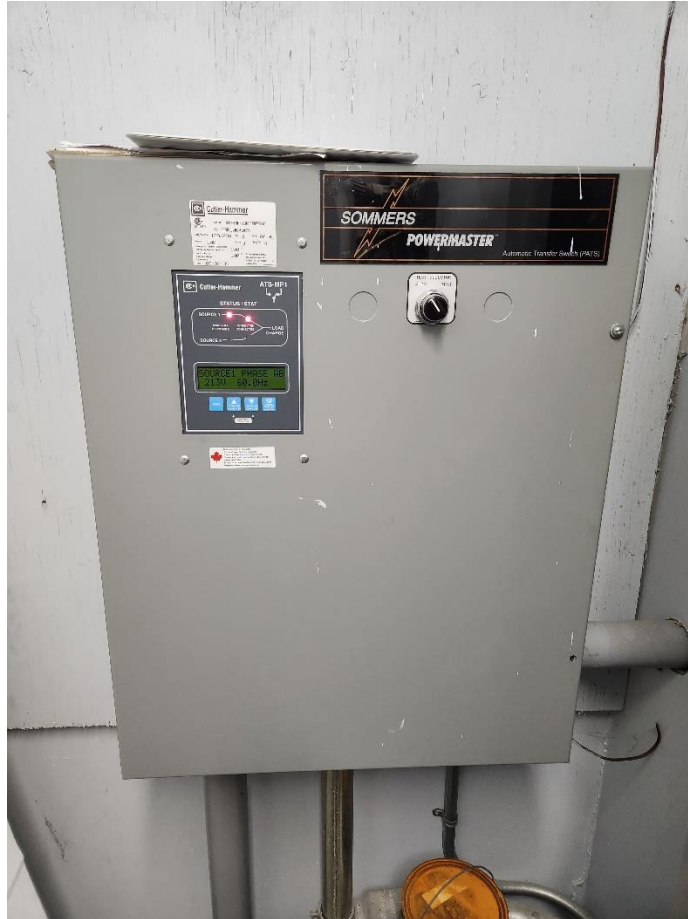
Photograph # 19 Automatic Transfer Switch
