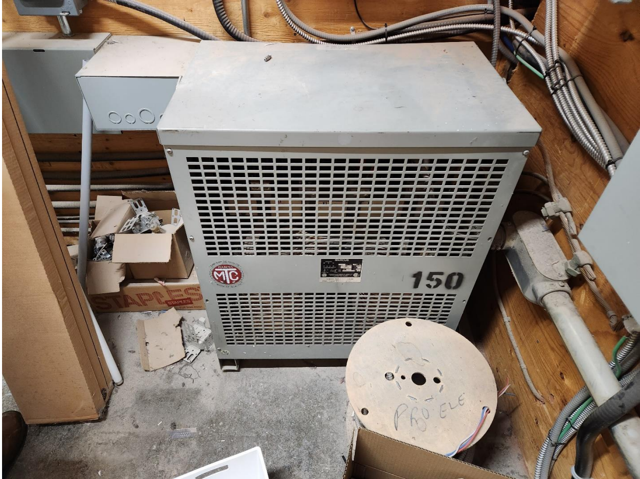
Photograph # 56 150 kVA Transformer
