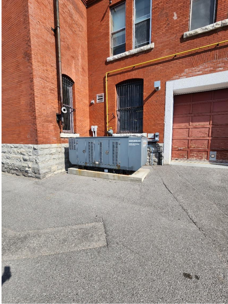
Photograph # 84 Backup Generator
