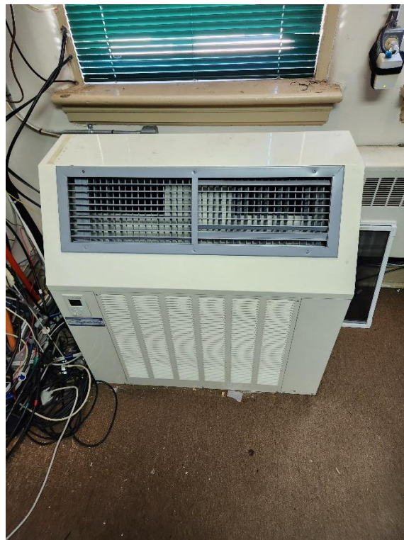
Photograph # 39 Floor AC Unit In IT Closet
