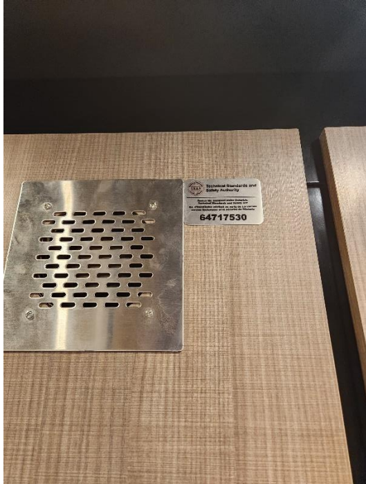
Photograph # 4 Elevator Safety Plate
