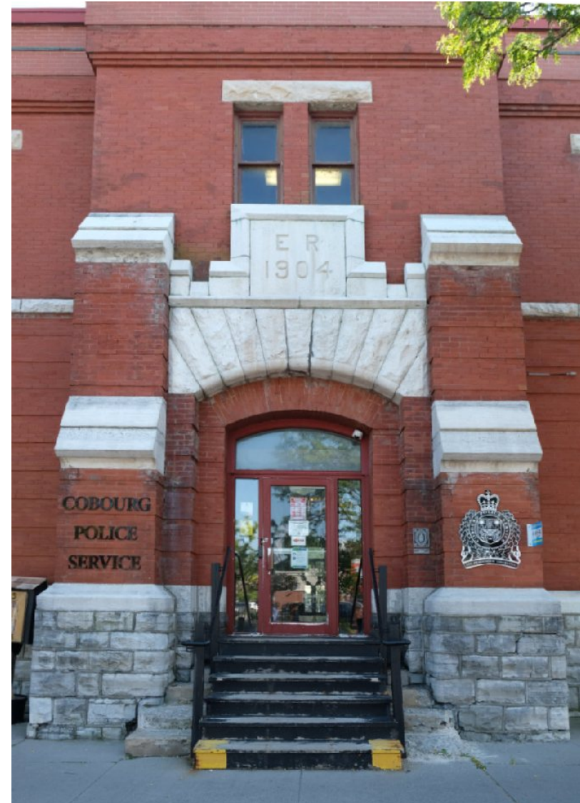
65. The current front entrance stair is severely deteriorate. a new wood stair to the entrance door has been built to allow access over the deteriorated stair. The existing door is a single leaf with sidelights and a single transom. Restoration of this important doorway and access stair is required. PGA
