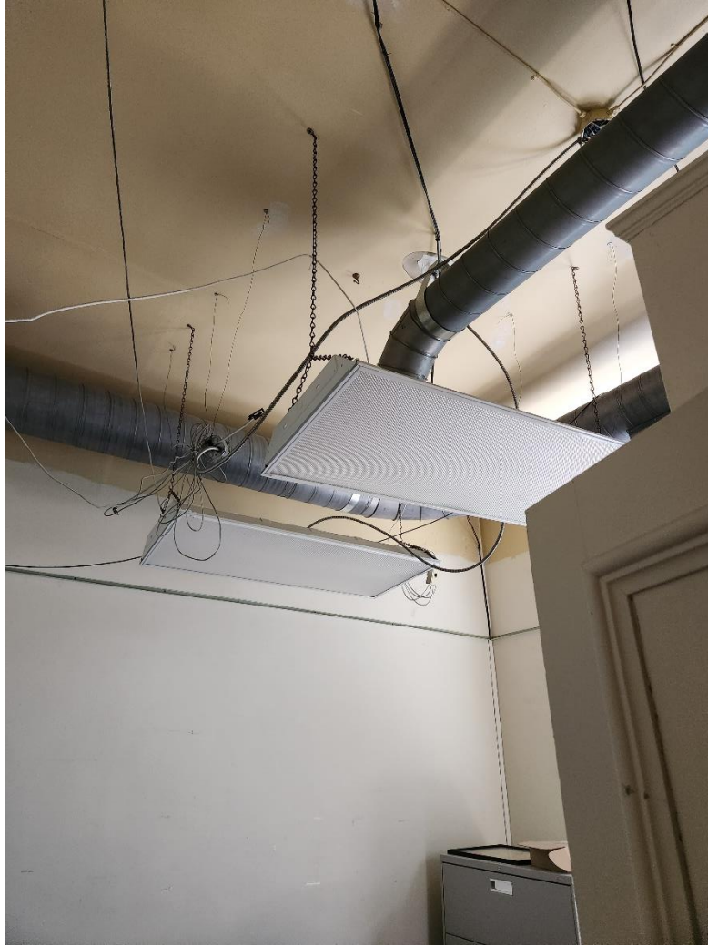
Photograph # 71 Ceiling Hung 2 by 4 Light Fixtures
