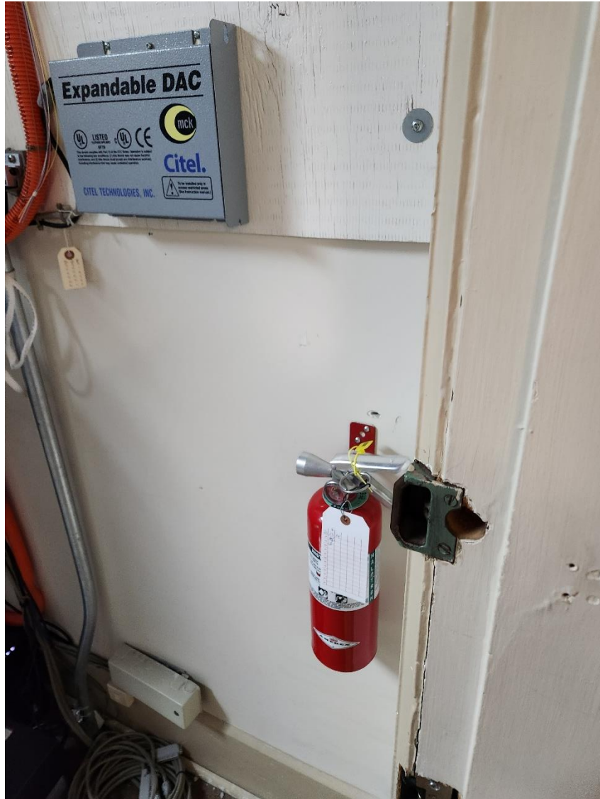
Photograph # 45 Fire Extinguisher
