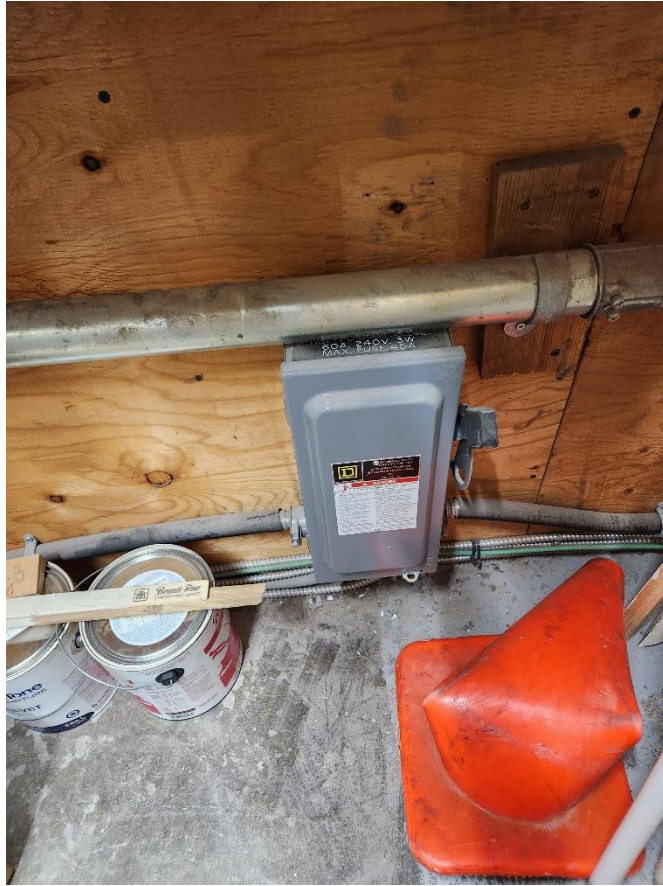
Photograph # 60 General Safety Switch
