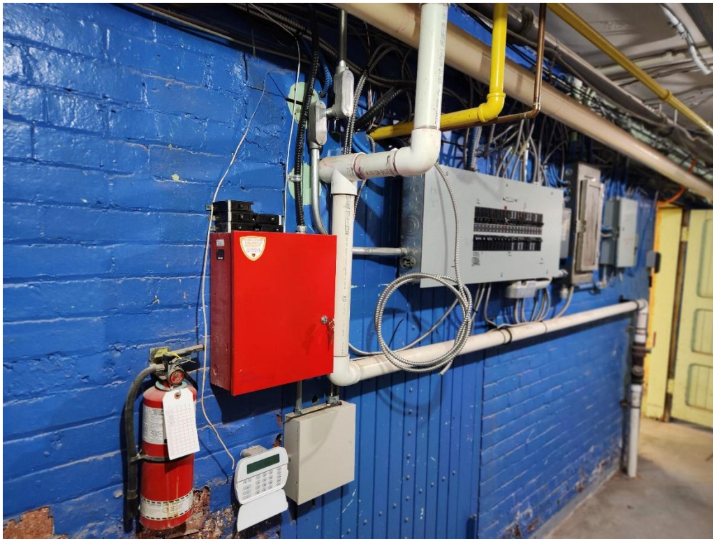
Photograph # 69 Fire Alarm Relay
