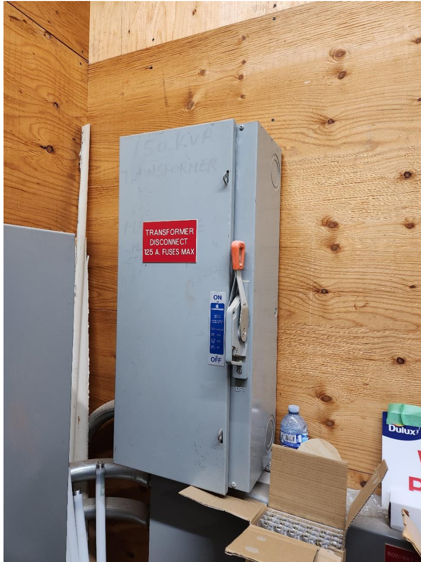
Photograph # 53 Transformer Disconnect
