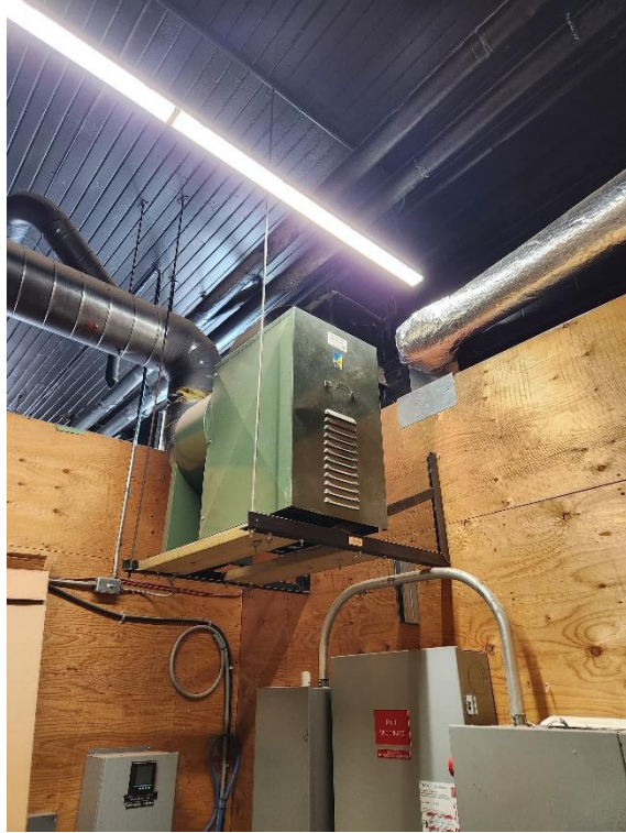
Photograph # 42 Electrical Room Power Ventilator
