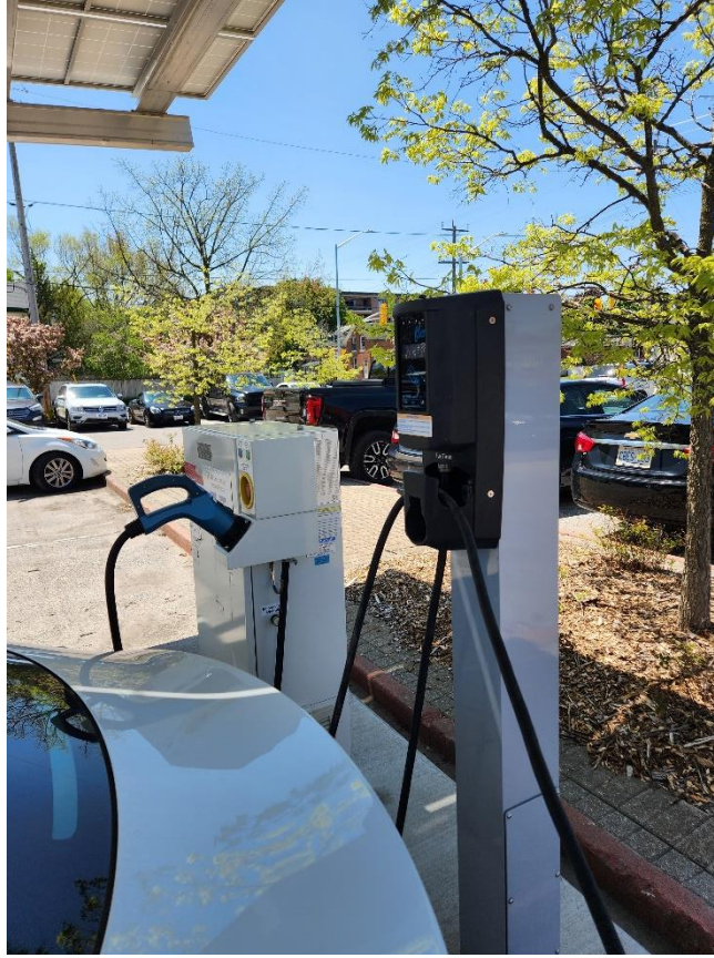
Photograph # 90 Level 3 EV Charger
