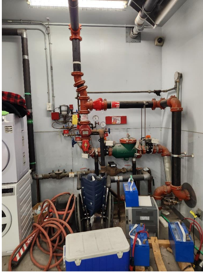
Photograph # 16 Sprinkler System Piping
