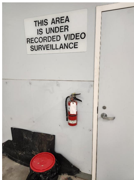
Photograph # 15 Fire Extinguisher
