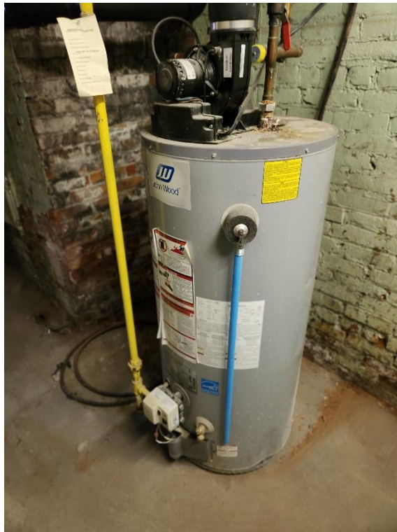
Photograph # 23 Natural Gas Hot Water Storage Tank
