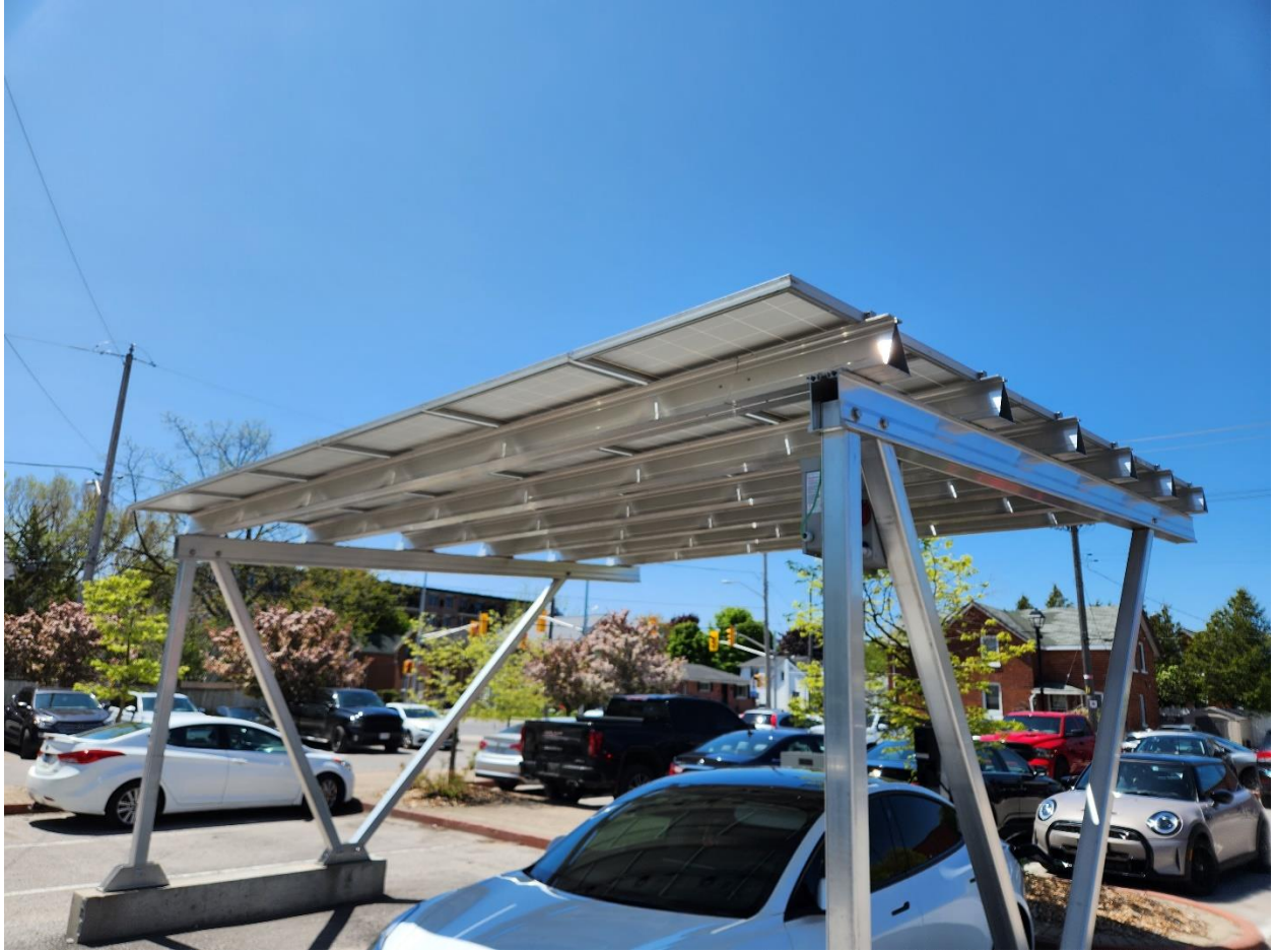
Photograph # 86 Solar PV Carport
