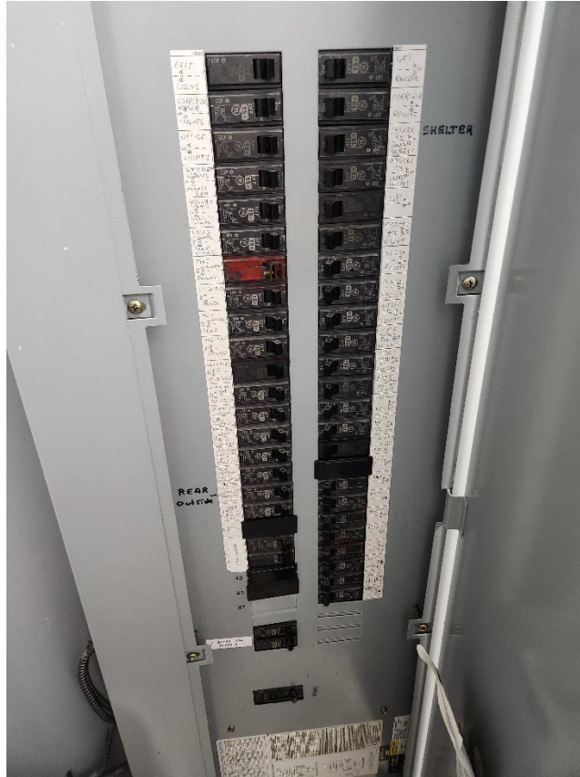
Photograph # 17 Main Distribution Panel
