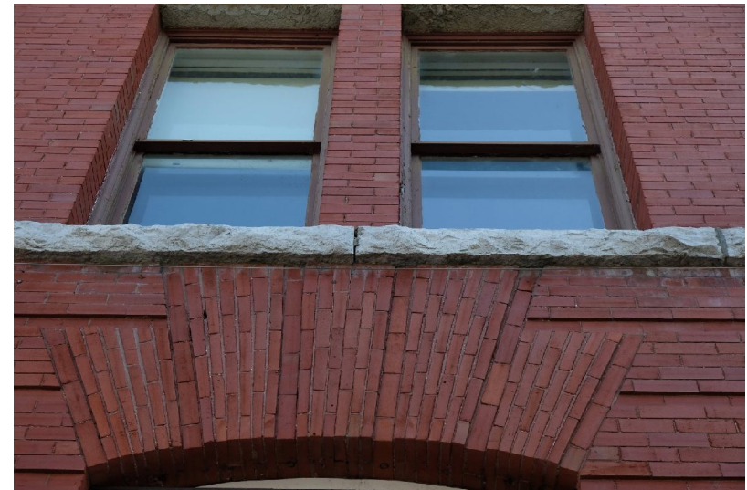
55. Detail of voussoir and second floor stone banding course-continuous sill. Note a number of open joints in both brick and stone. Many vertical joints in the banding course and some localized areas of brick walling require repointing. PGA
