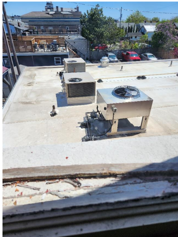
Photograph # 9 Rooftop Dual Heating Cooling Units
