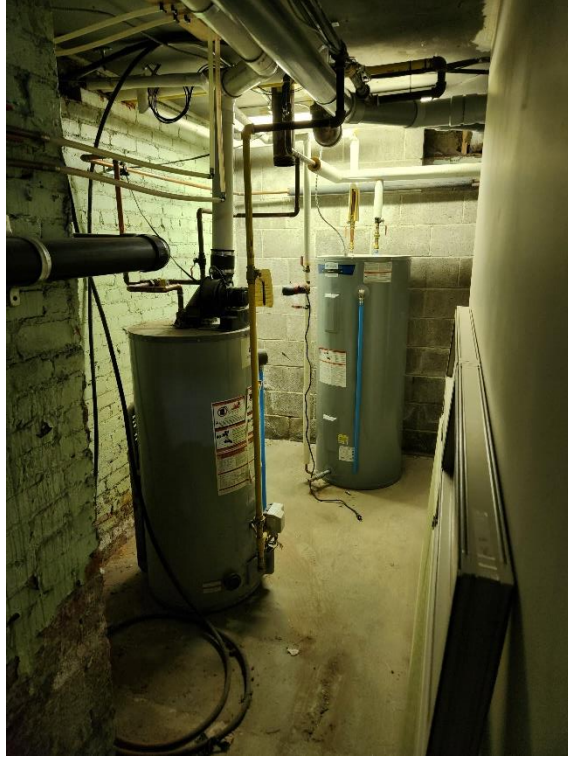
Photograph # 22 Hot Water Storage Tanks
