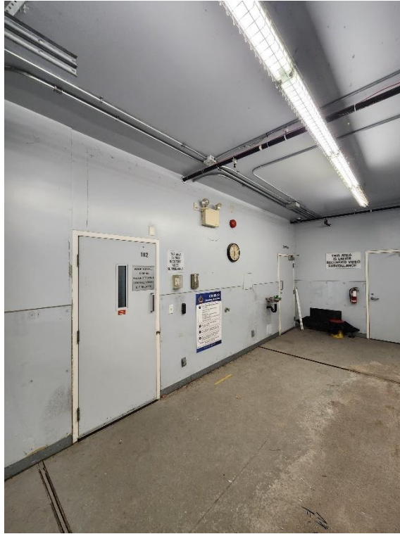
Photograph # 23 T5 Caged 2 Lamp Fluorescent Light Fixtures
