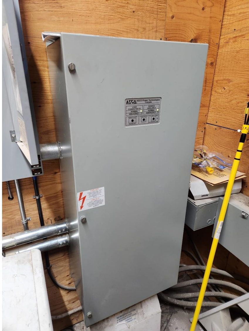
Photograph # 59 ASCO Power Automatic Transfer Switch
