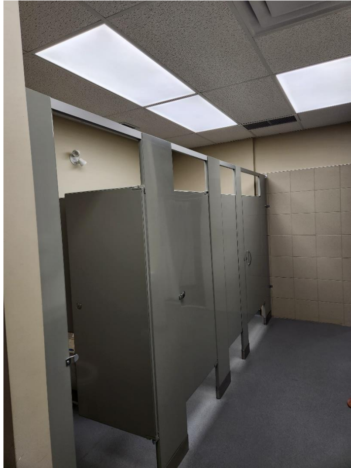
Photograph # 76 2 by 4 Light Fixtures in Women's Changeroom
