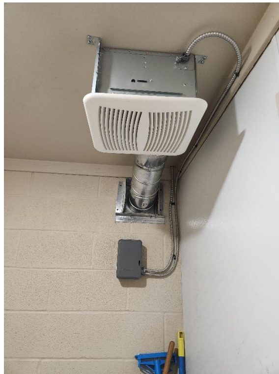
Photograph # 41 Janitorial Closet Exhaust Fan
