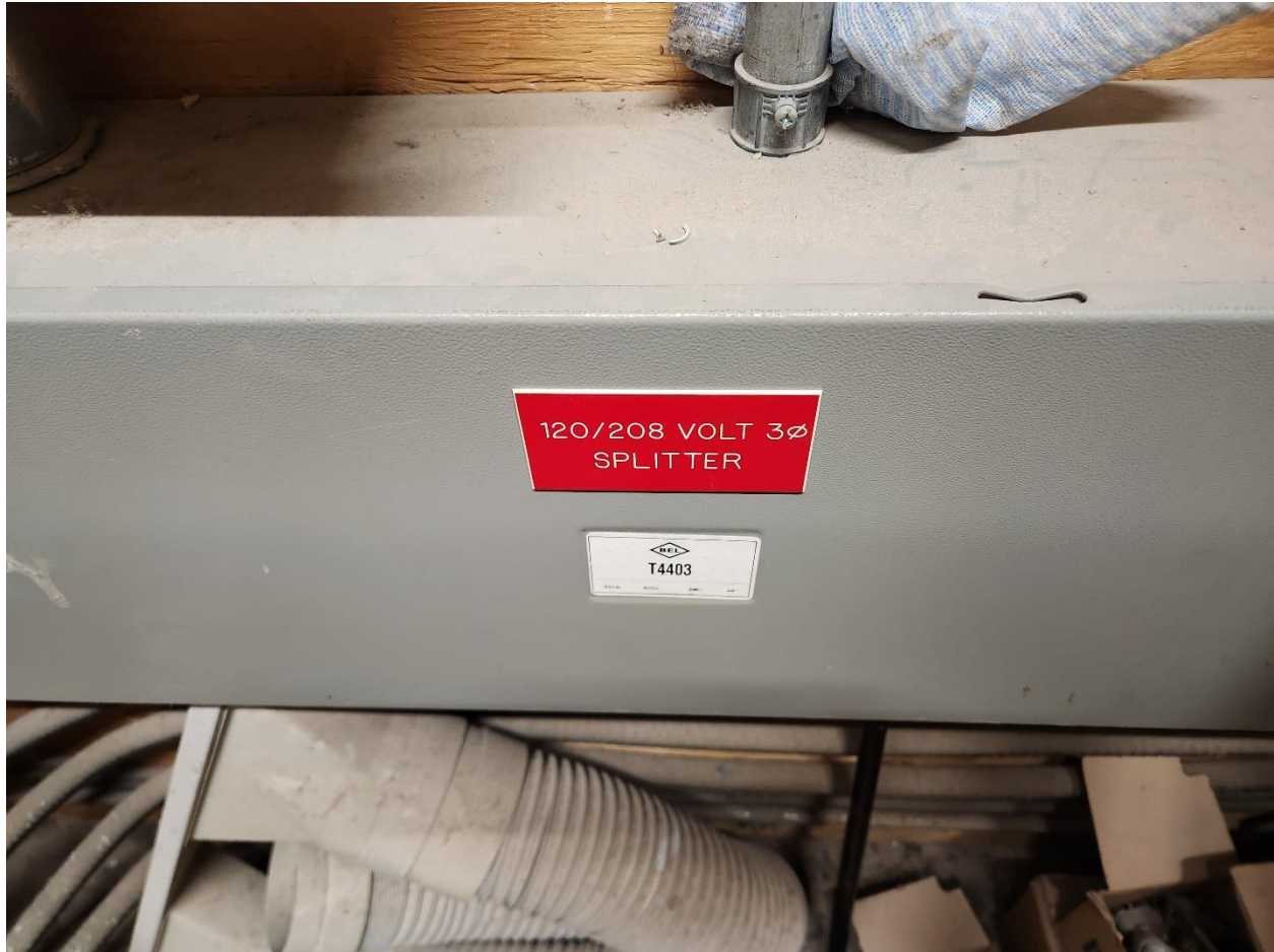
Photograph # 58 120/208V Splitter
