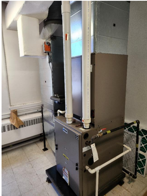
Photograph # 28 York Natural Gas Furnace
