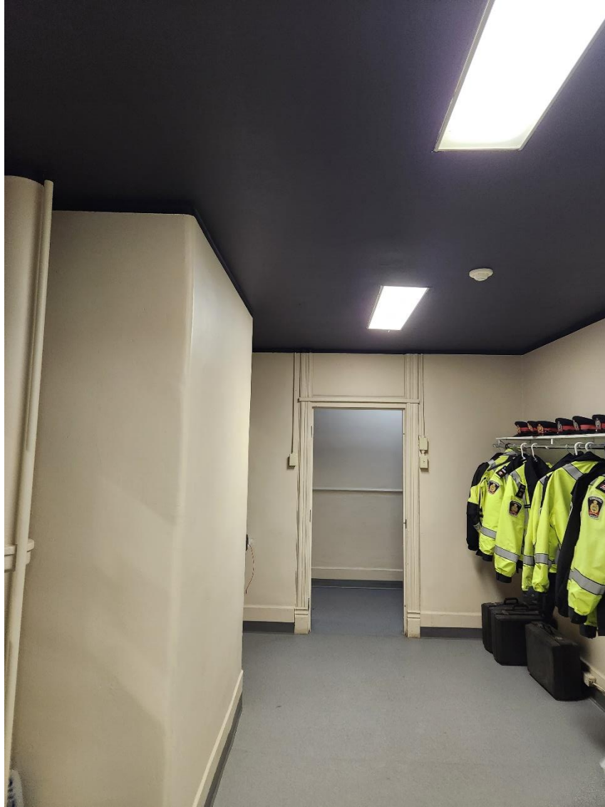
Photograph # 75 1 by 4 Ceiling Mounted Lights
