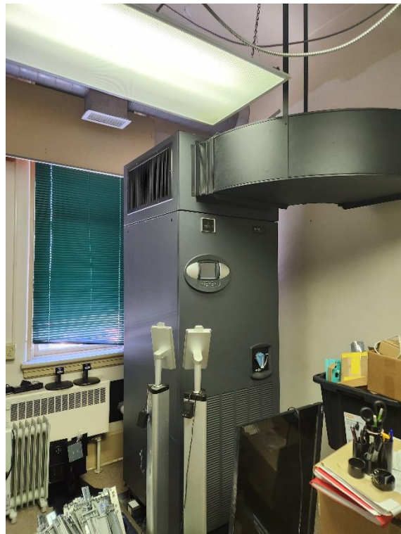
Photograph # 37 CRAC Unit in IT Closet
