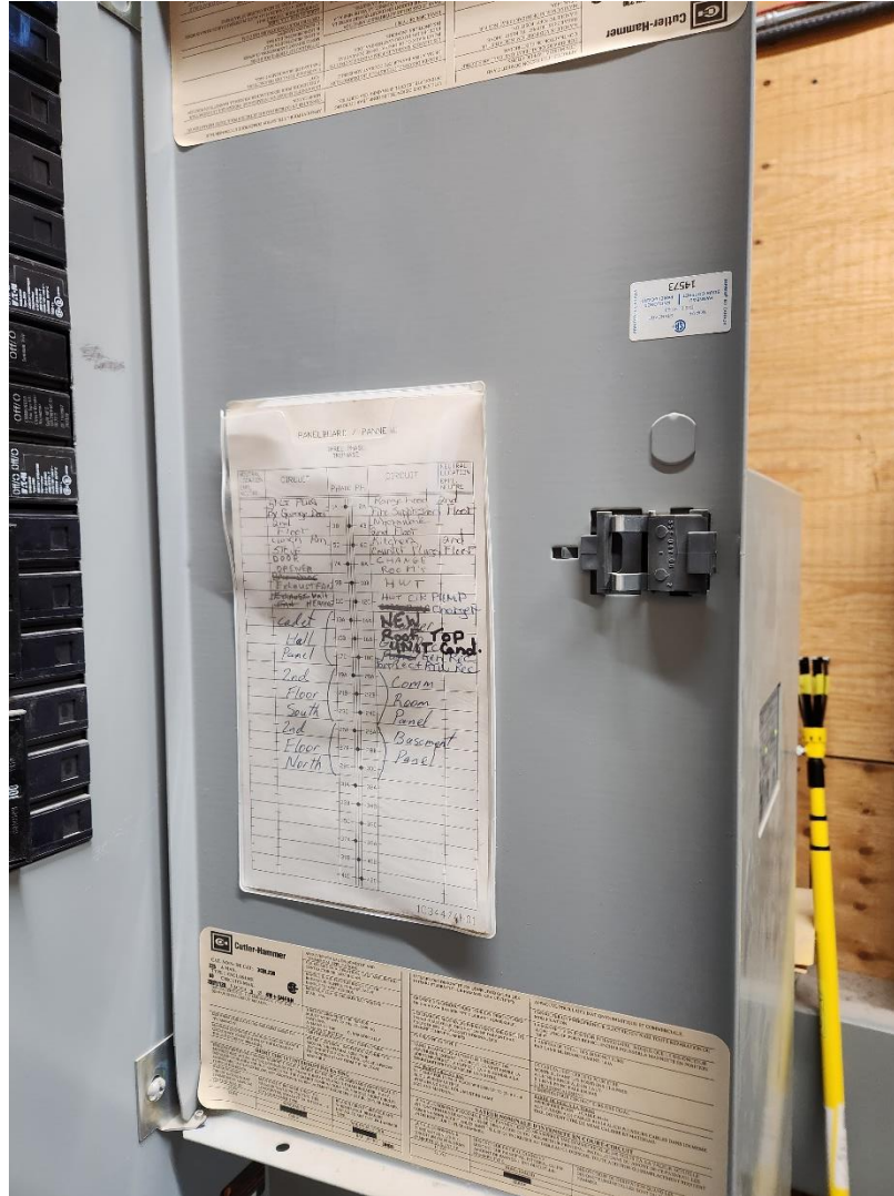
Photograph # 47 Main Distribution Panel Nameplate
