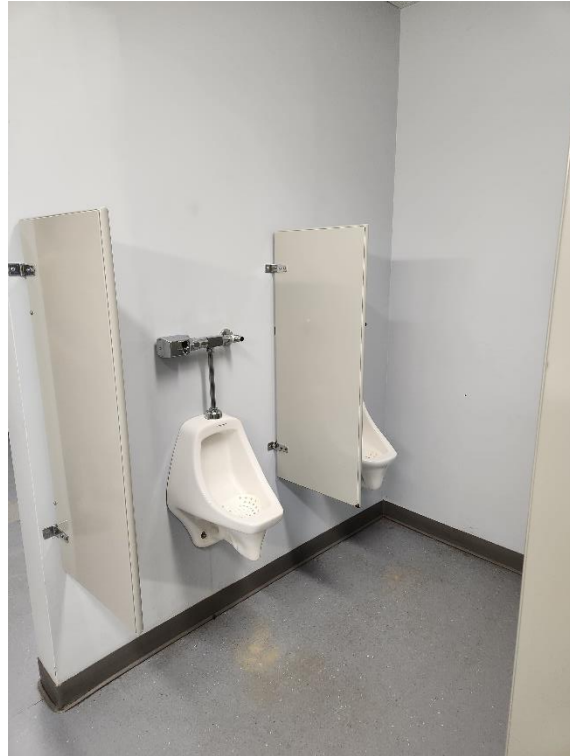
Photograph # 7 Men's Changeroom Urinals
