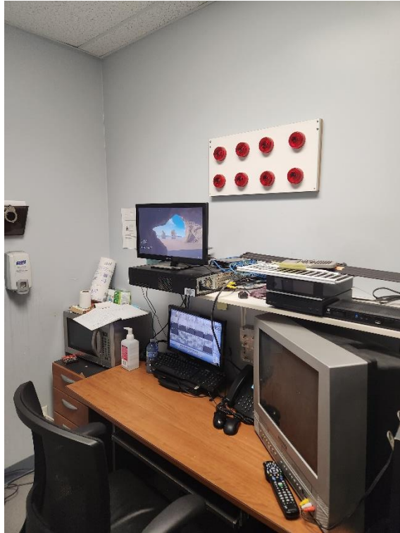
Photograph # 25 IT room
