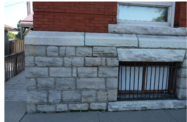
51. Similar to above, note some settlement in the foundation and resulting cracking largely at joints between stone units as well as vertical joints in the banding course. All open joints should be repointed. PGA
