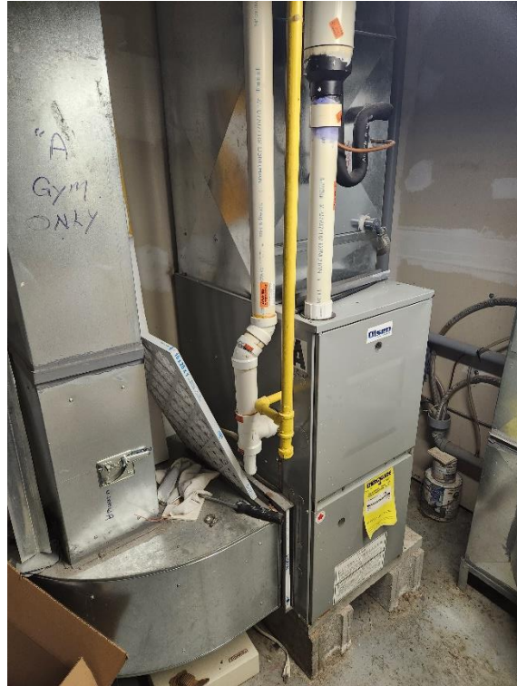
Photograph # 30 Olsen Natural Gas Furnace
