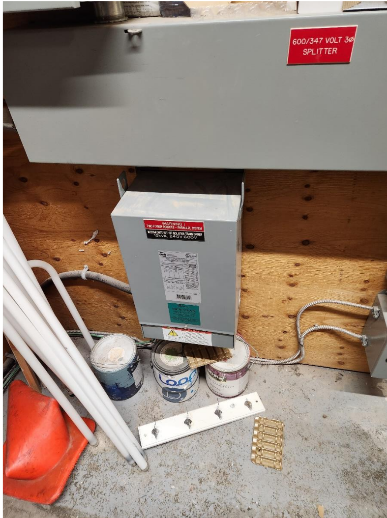
Photograph # 63 15 kVA Transformer
