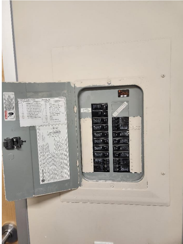
Photograph # 65 First Floor Electrical Panel
