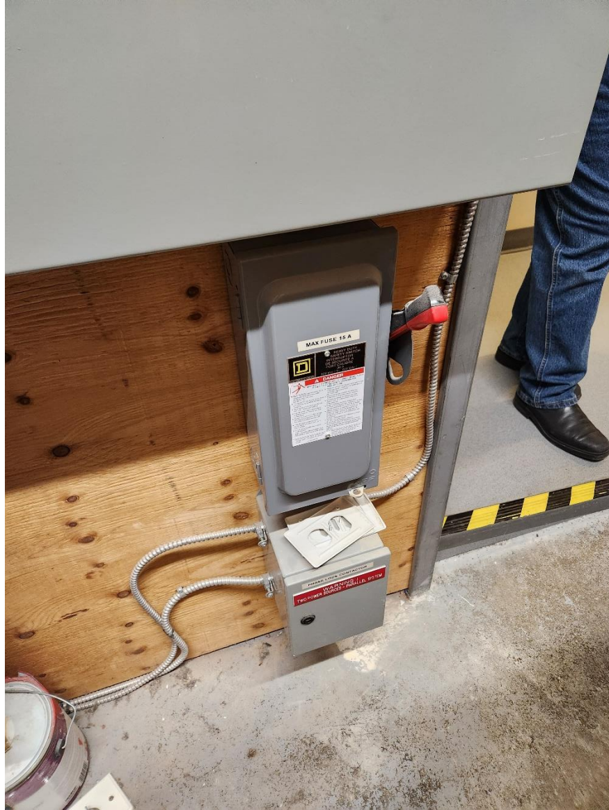
Photograph # 62 Heavy Duty Safety Switch and Phase Loss Monitor
