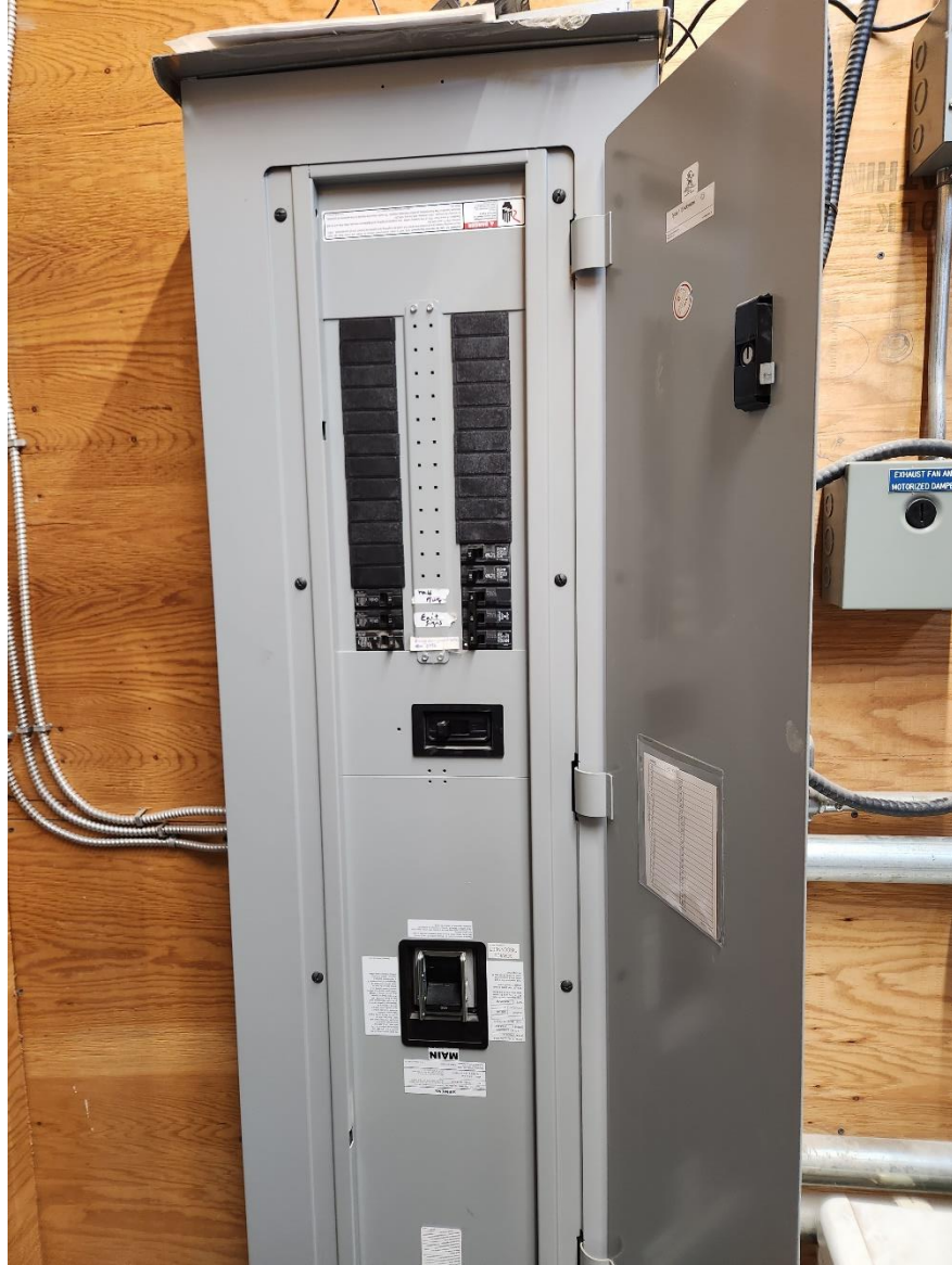
Photograph # 48 Main Disconnect Panel
