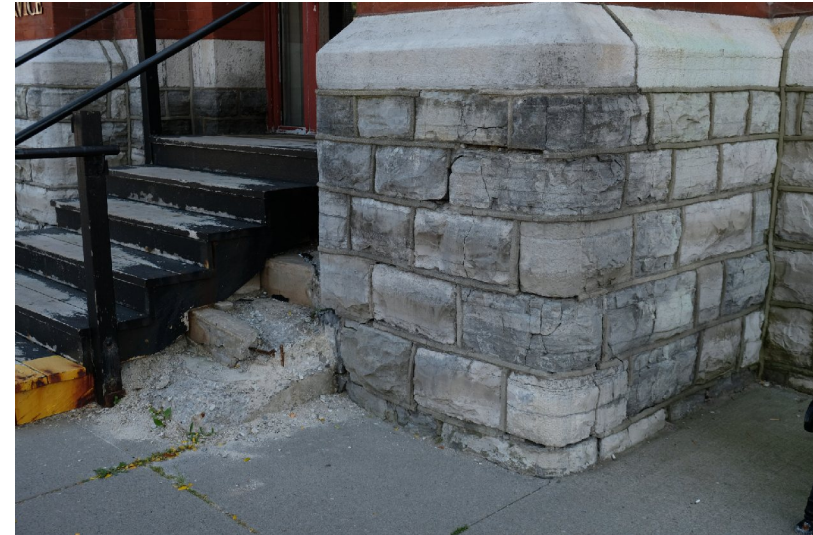
66. Detail view at the existing front stair, the scope of deterioration in this area is clearly illustrated. PGA
