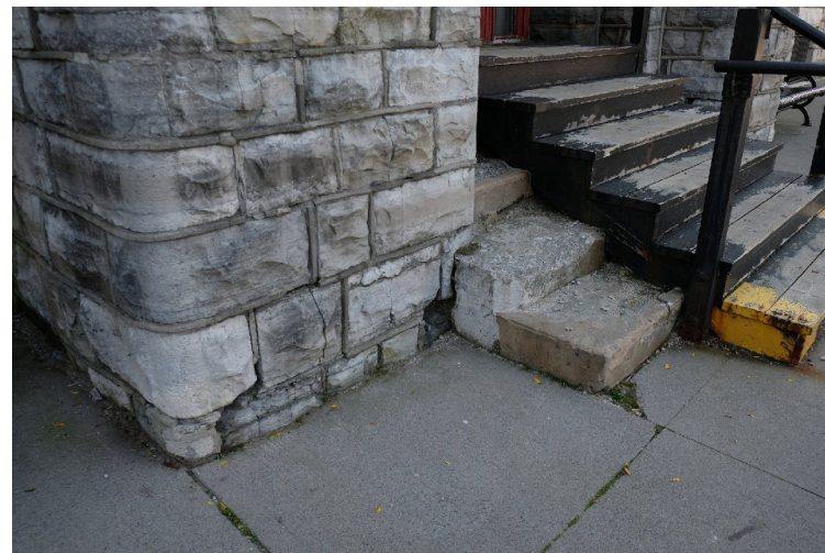
47. Detail view of the north-east corner of entrance bay, This wall has also shifted and lower joints and some stone units are deteriorated, from the use of salt. The entire foundation and stair assembly of the front entrance requires repairs. PGA
