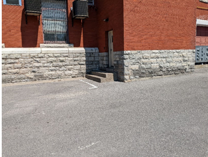
Picture 1: Picture taken from the back of building toward the Exist. Exit from the building is not level to the ground level.
