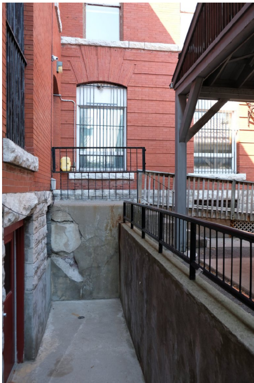
50. Left. Basement entrance at the east side. Ramps provide accessibility into the building as seen here. The foundation of the upper ramp is severely deteriorated and requires repair. PGA
