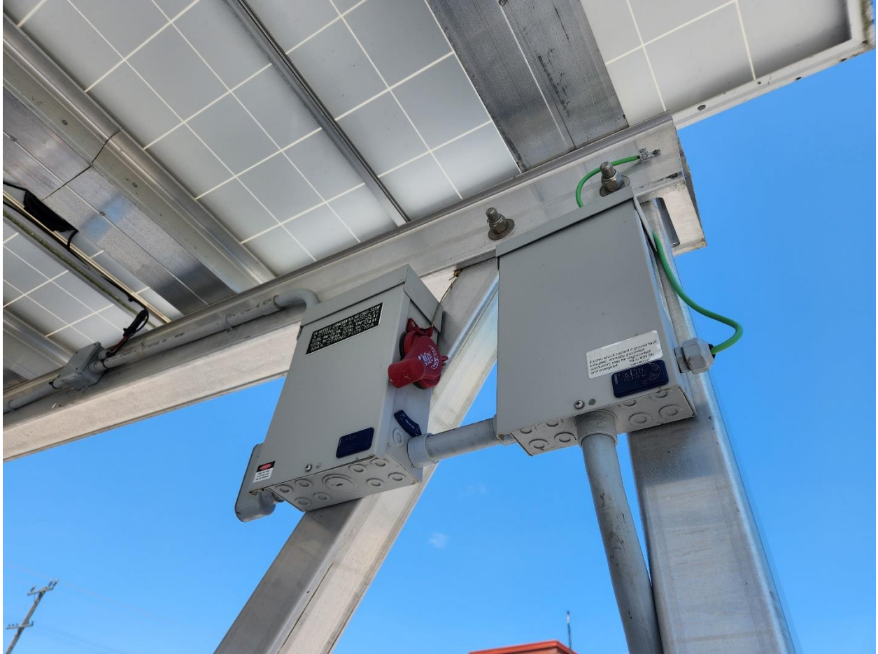
Photograph # 87 PV Module
