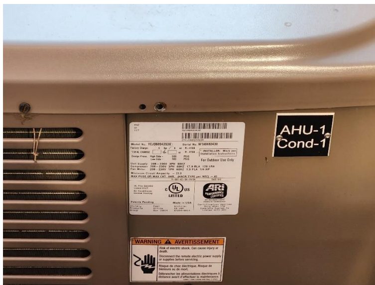
Photograph # 35 York Condenser Unit Nameplate
