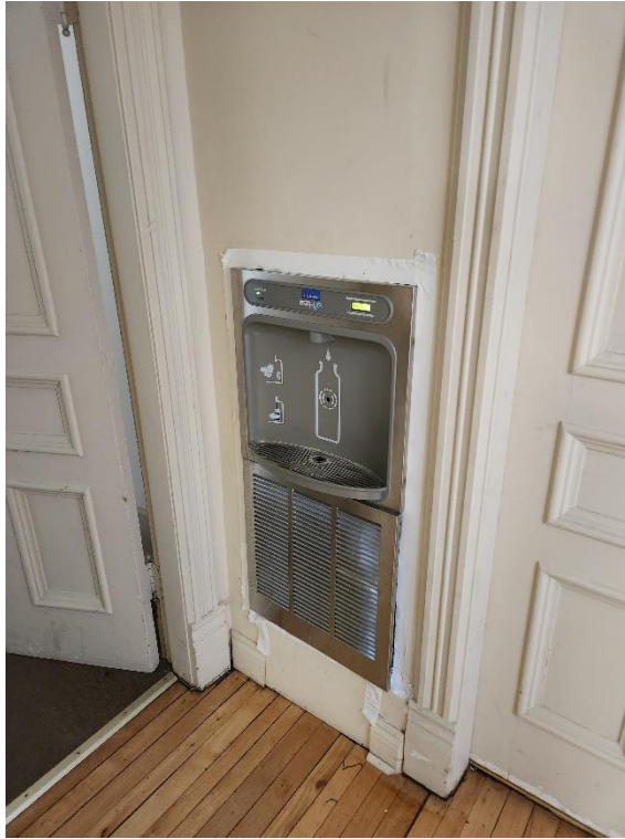
Photograph # 20 Water Bottle Refill Station
