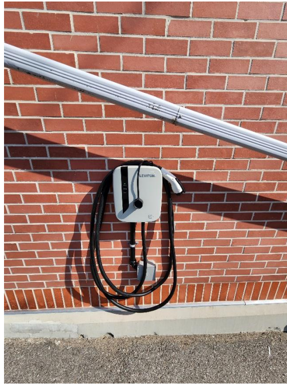
Photograph # 28 Level 2 EV Charger
