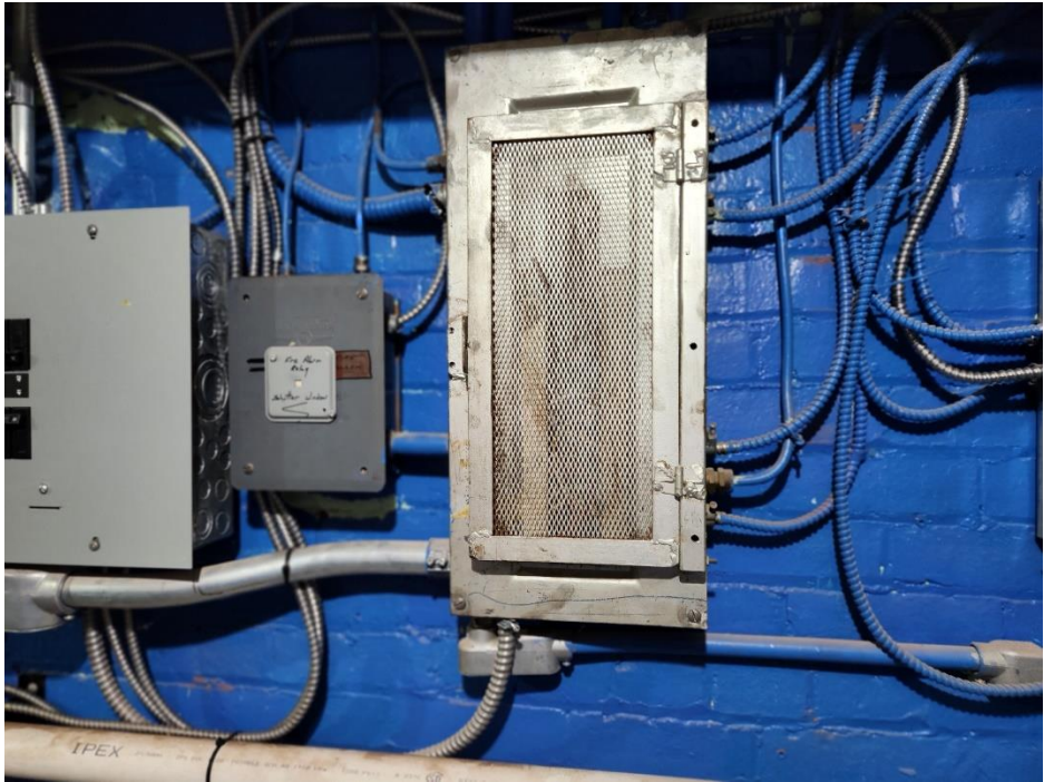
Photograph # 68 Small Electrical Panel in Basement
