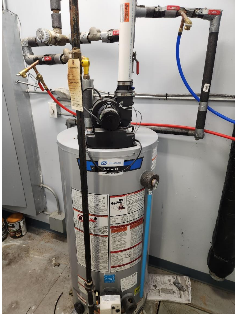
Photograph # 7 Natural Gas Hot Water Storage Tank
