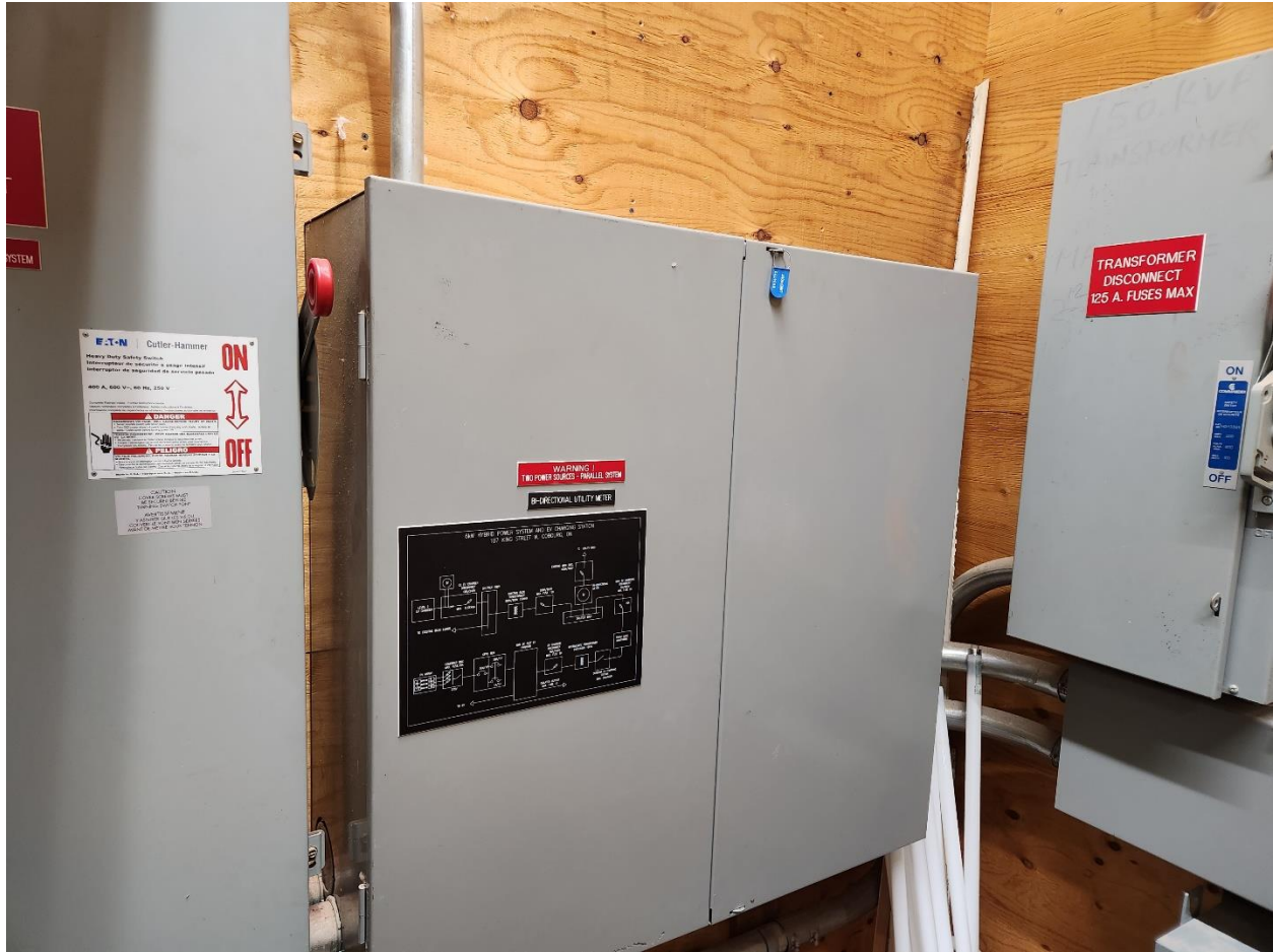
Photograph # 50 Bi-Directional Utility Meter
