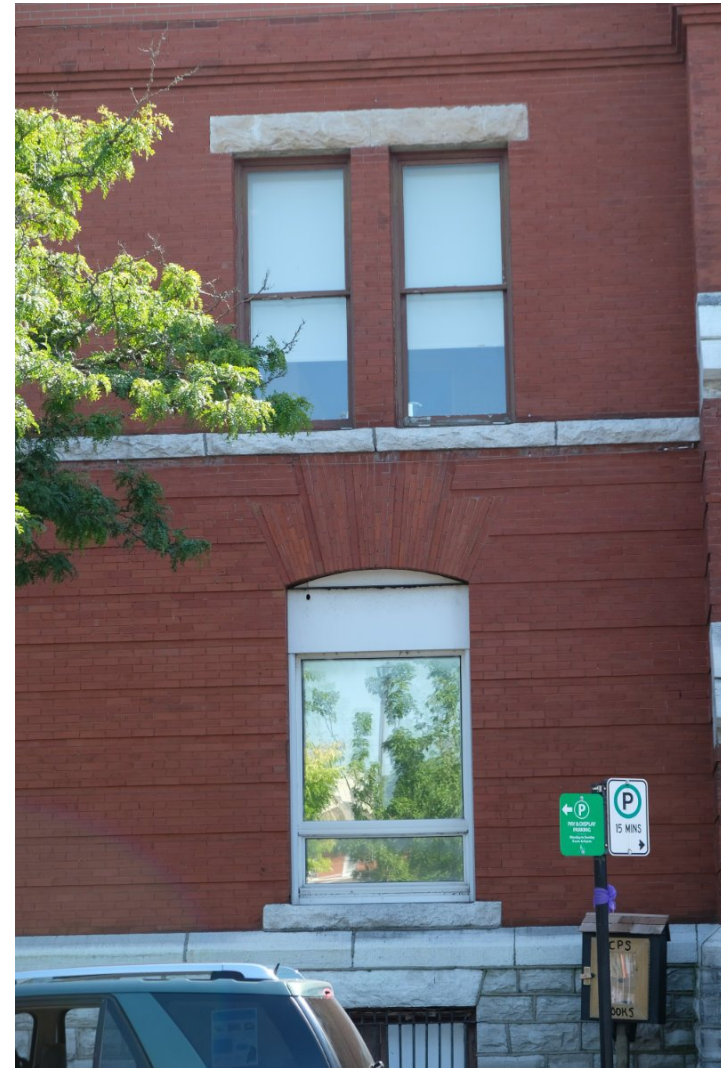
57. View of windows on the north elevation east. The upper 1/1 wood windows are original the lower window has been replaced with an ill fitting smaller aluminium window and solid transom within the original window opening. PGA
