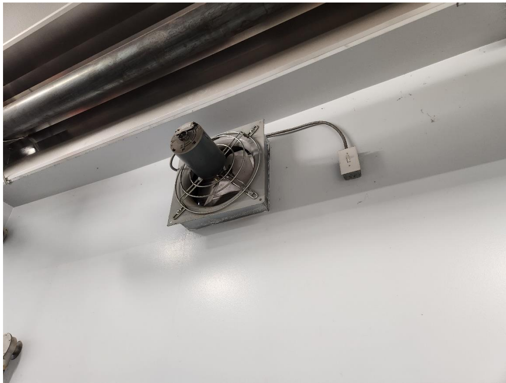
Photograph # 13 Garage Exhaust Fan and Switch Controller
