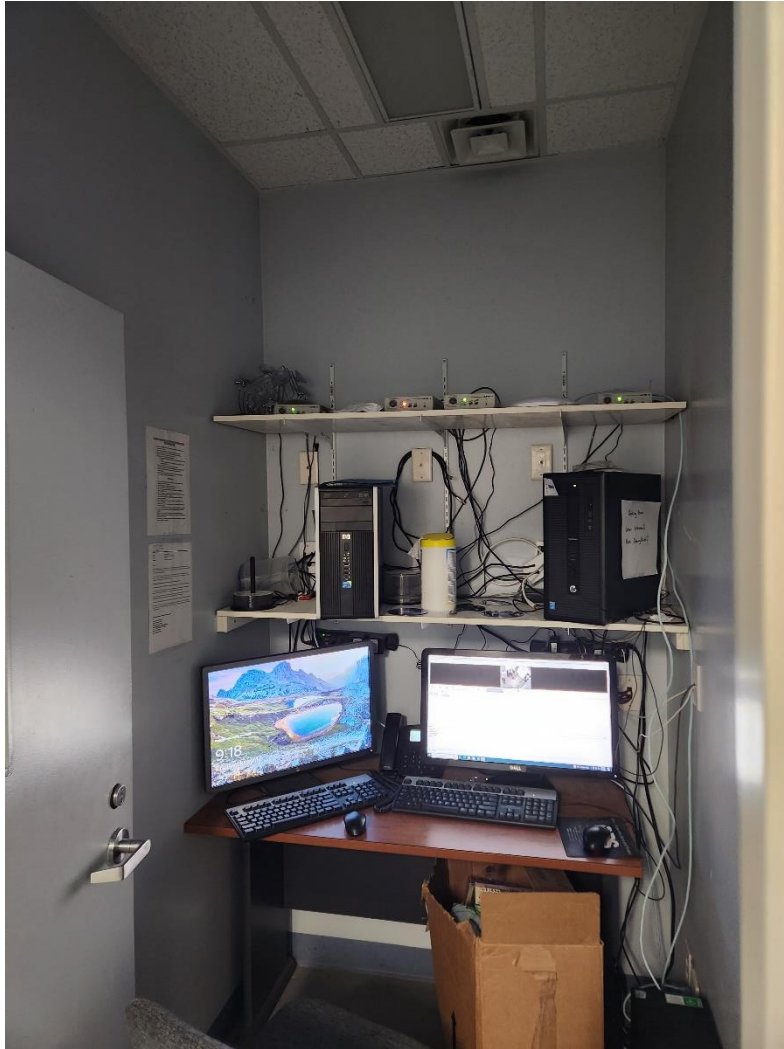
Photograph # 27 Security Surveillance Room
