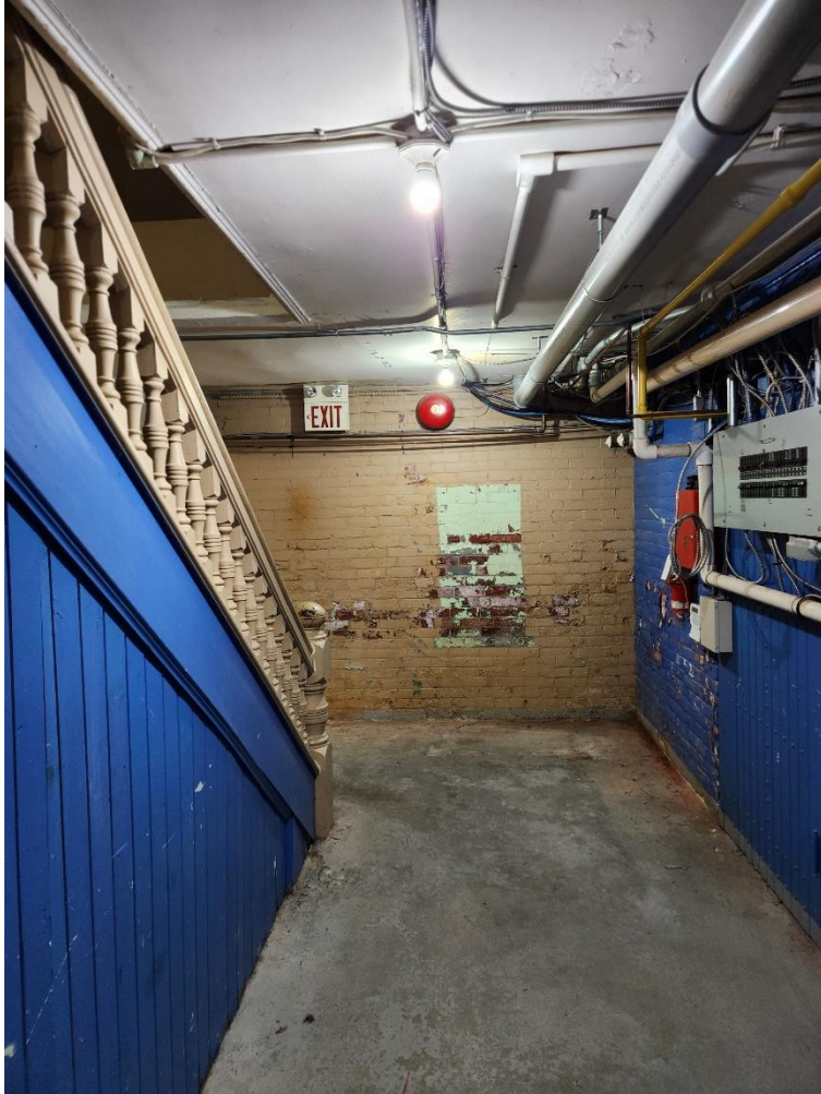
Photograph # 70 A19 Single Bulb Fixtures
