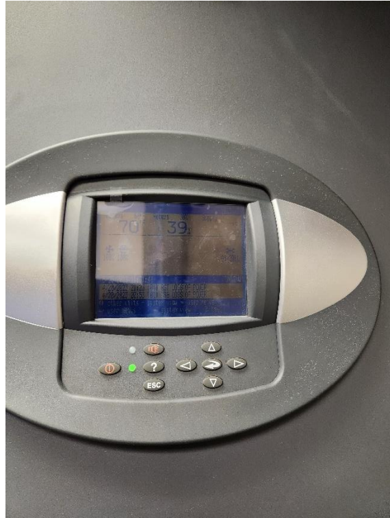
Photograph # 38 CRAC Unit Controller
