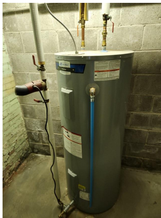
Photograph # 25 Electric Hot Water Storage Tank
