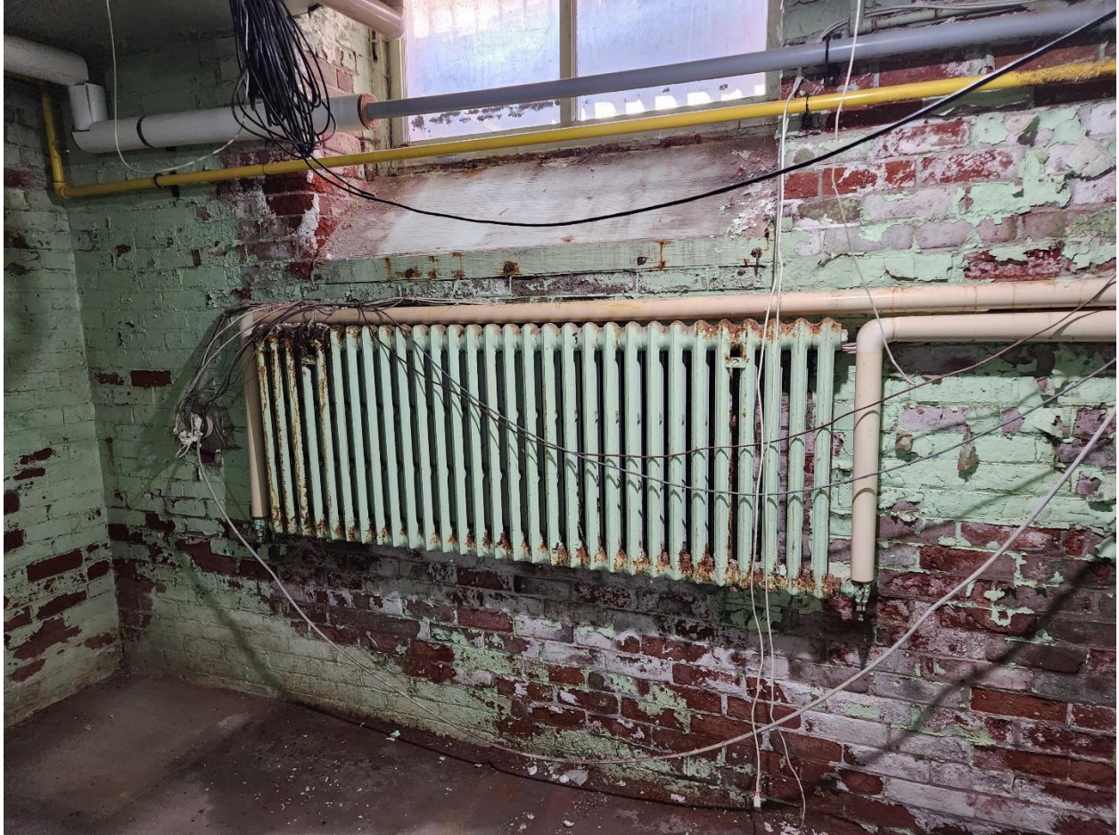
Photograph # 32 Abandoned Radiator
