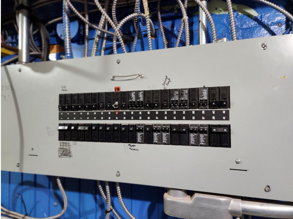
Photograph # 67 Large Electrical Panel in Basement
