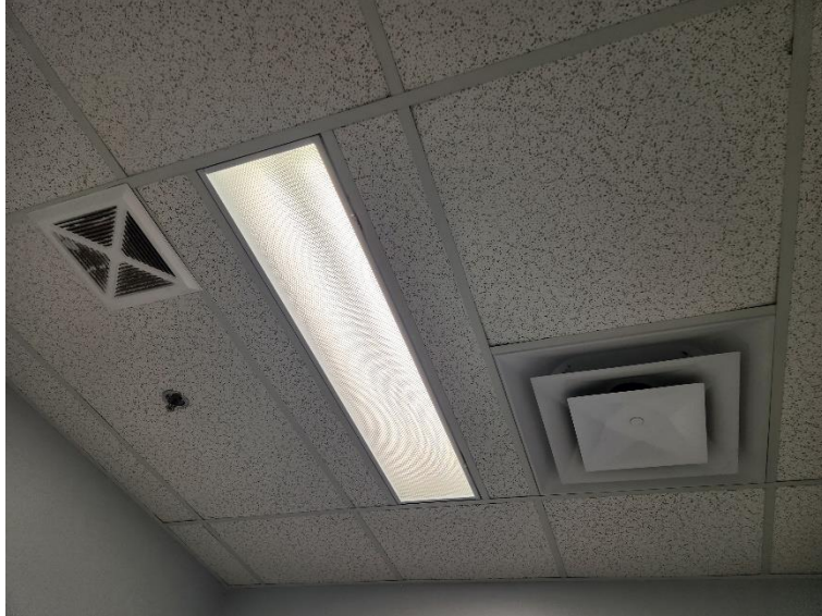
Photograph # 12 1 by 4 Light Fixture and Ductwork Diffuser
