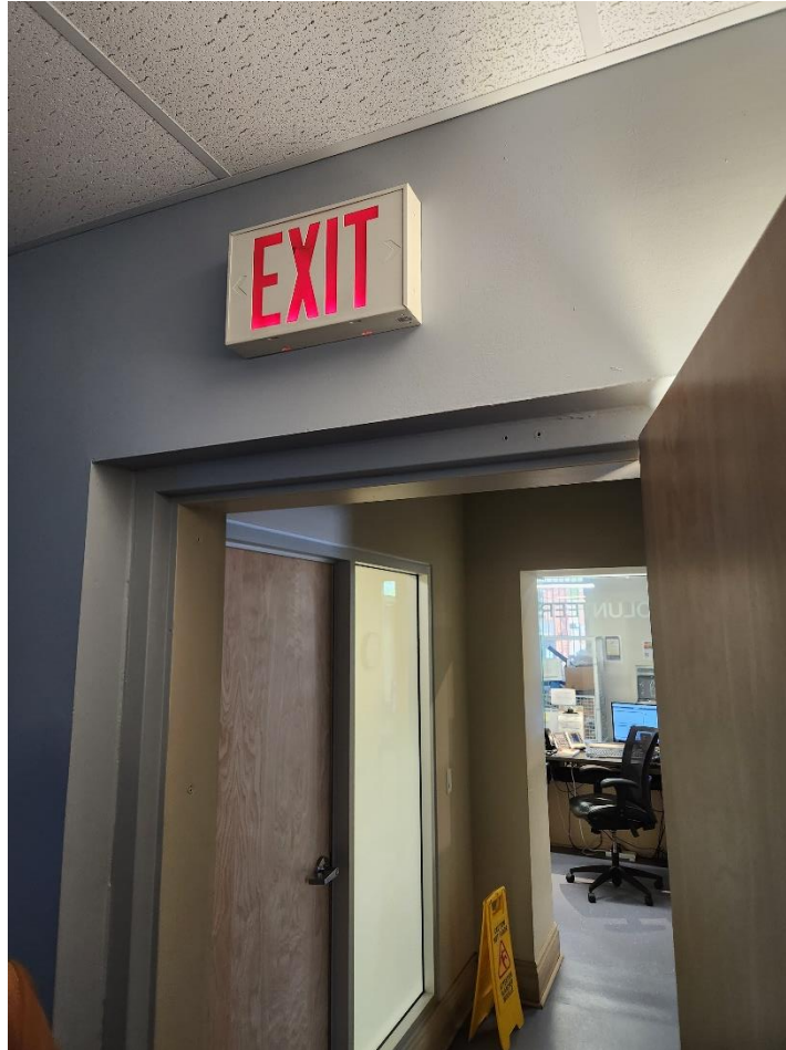
Photograph # 79 Red Exit Sign
