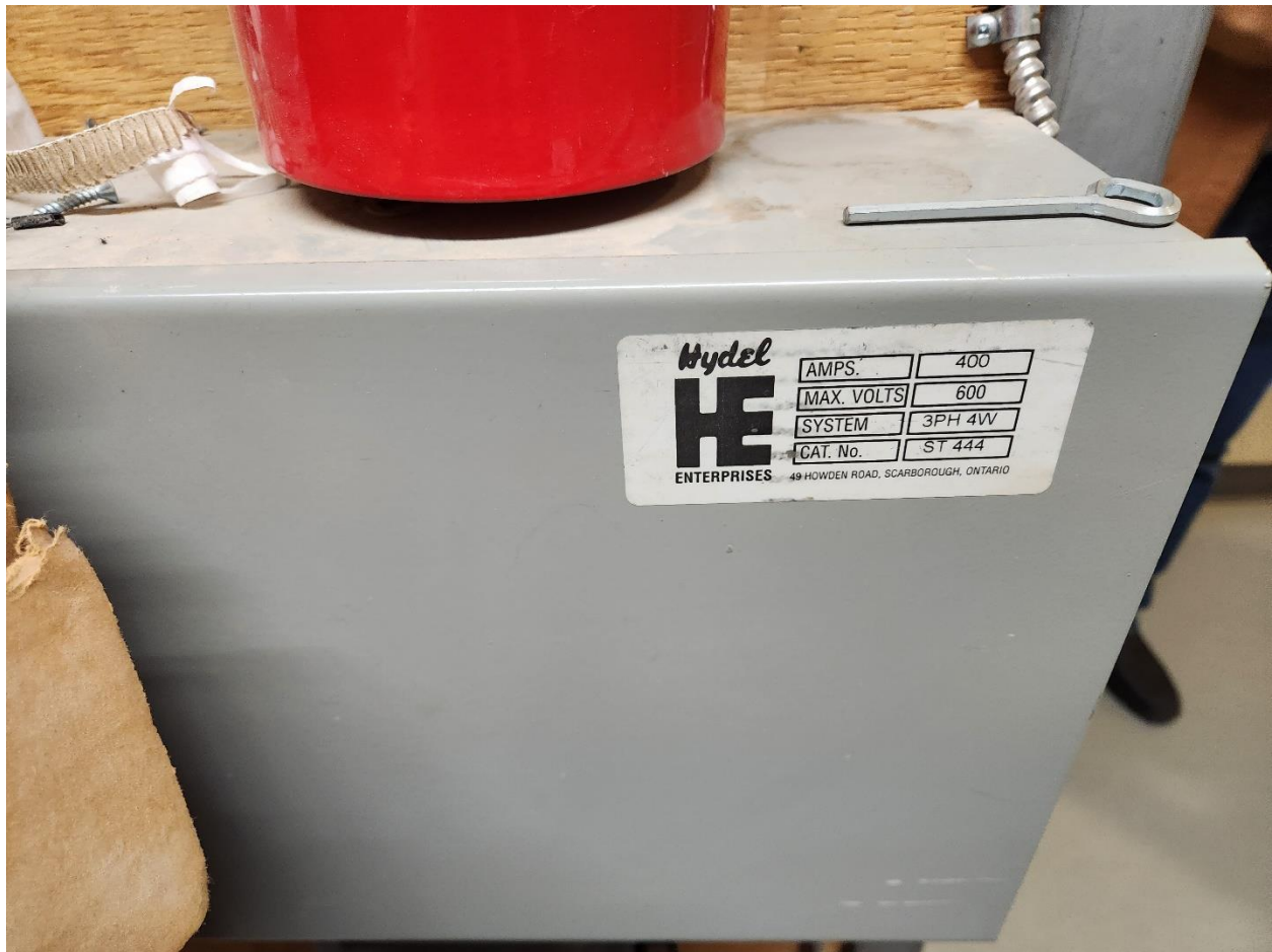
Photograph # 52 High Voltage Splitter Nameplate
