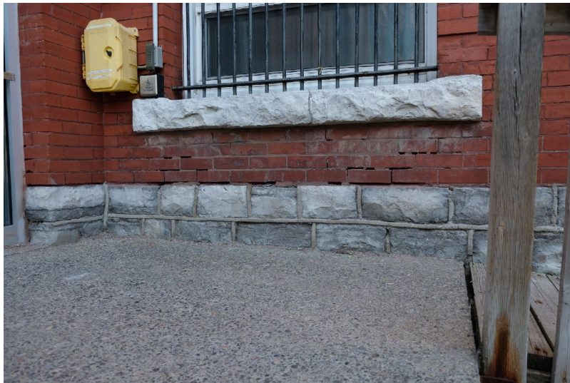
54. A cracked sill and open joints are allowing water into the wall resulting in staining through lime migration. All open joints should be repointed to prevent further deterioration. repointing. PGA
