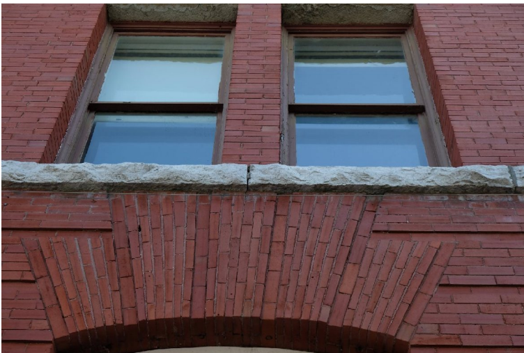
60. View to second floor window showing the detailed decorative brick voussoir over the ground floor windows . PGA
