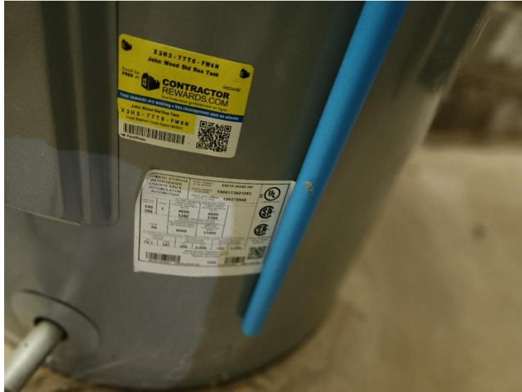
Photograph # 26 Electric Hot Water Storage Tank Nameplate
