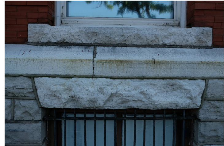
49. View of lug sill at first floor window and dressed banding above the rusticated foundation. Many vertical joints in the banding course and sills where they exist require repointing. PGA
