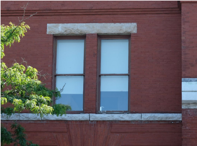
58. Second floor windows are paired 1/1 wood windows separated by a brick pier. All wood windows require attention, putty, filling, sanding scraping and repainting, and may require cord replacements for functionality of required to open. PGA
