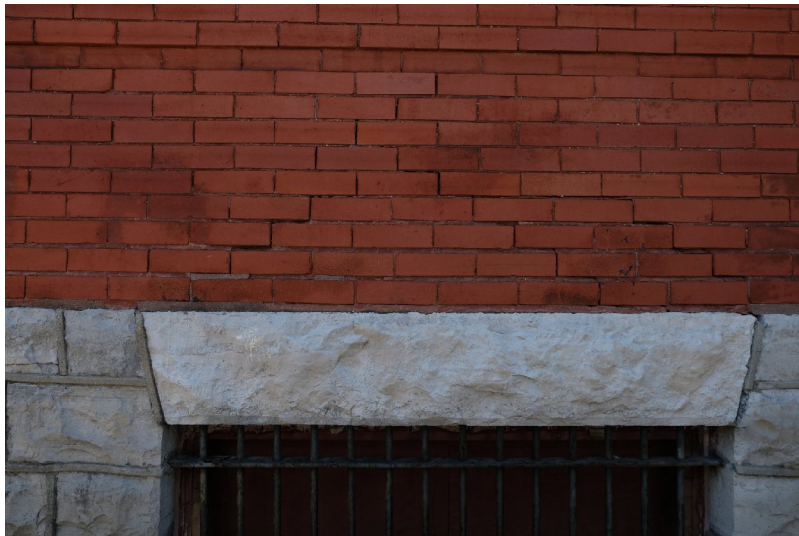
56. This basement stone lintel has shifted as joints deteriorate allowing a prism of brick to drop. Note stepped cracking at brick joints. PGA
