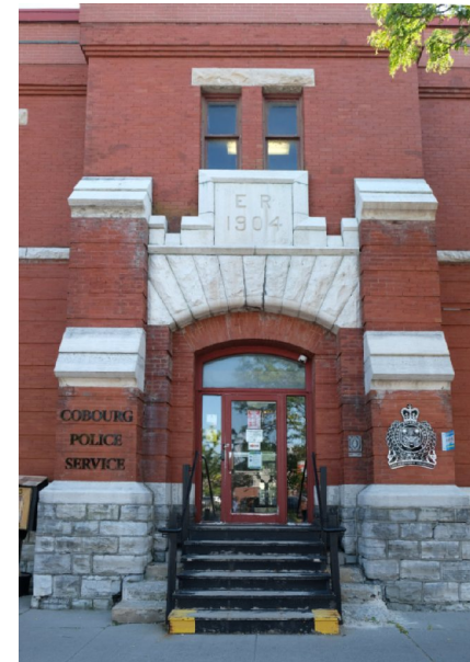
45. View of the front entrance bay on King St. The raised parapet has been altered. The front stairs are severely deteriorated and overbuilt with a wood stair for access. The entrance door has been replaced. PGA
