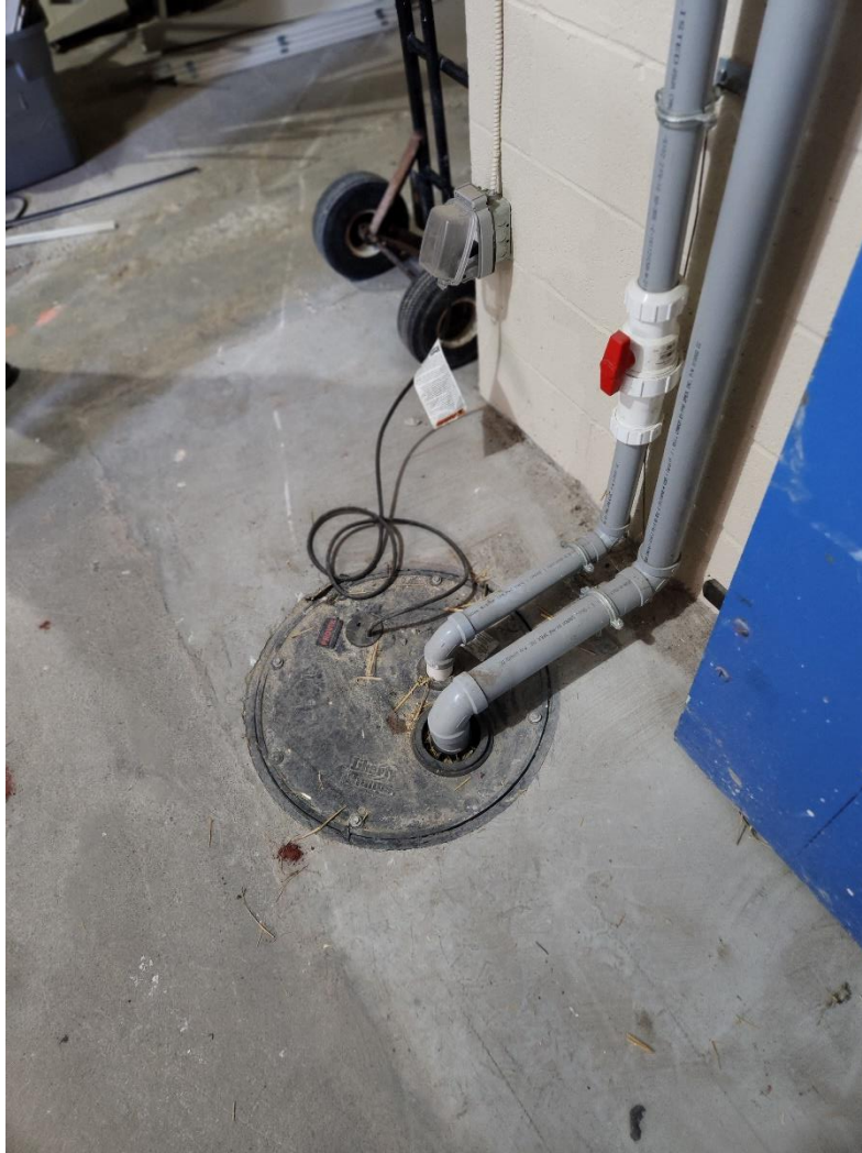
Photograph # 27 Outgoing Sewer to sump pump pit
