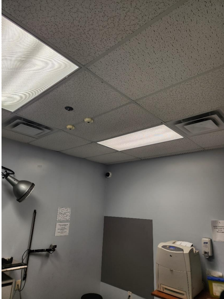
Photograph # 21 2 by 4 Light Fixtures
