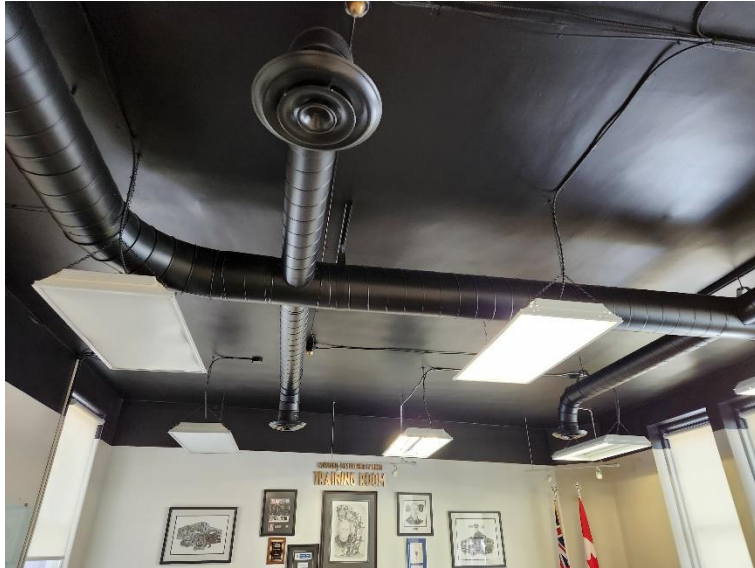
Photograph # 40 Metal Ductwork and Diffusers
