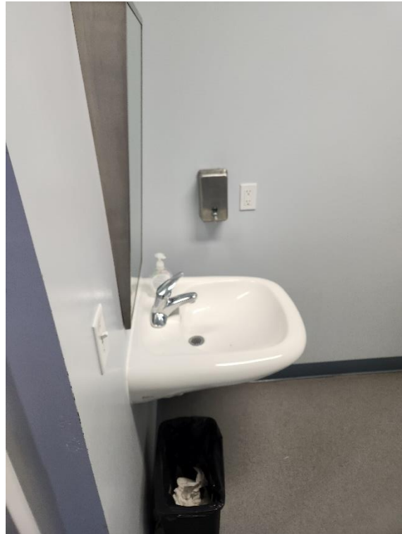
Photograph # 5 Washroom Sink
