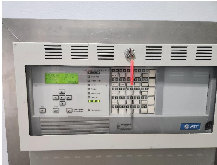
Photograph # 24 Fire Alarm System Panel
