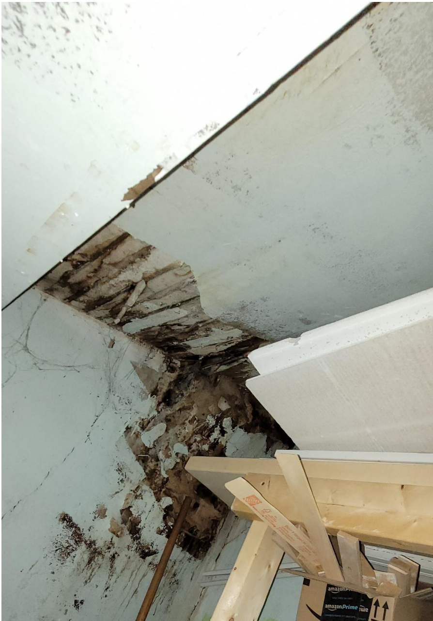
Figure 6: 36 King St. W – photo showing roof leak damage on the interior – black mould?
