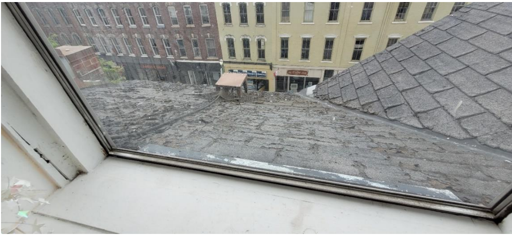
Figure 1: 36 King St. W – current condition of a portion of the roof
