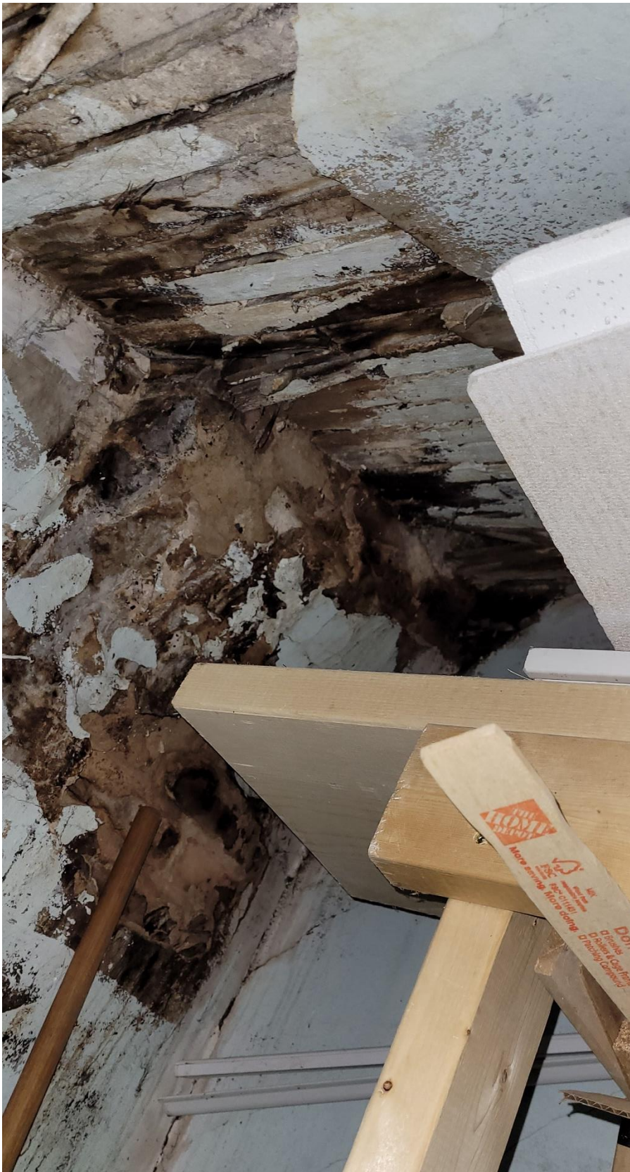
Figure 5: 36 King St. W – photo showing roof leak damage on the interior – black mould?
