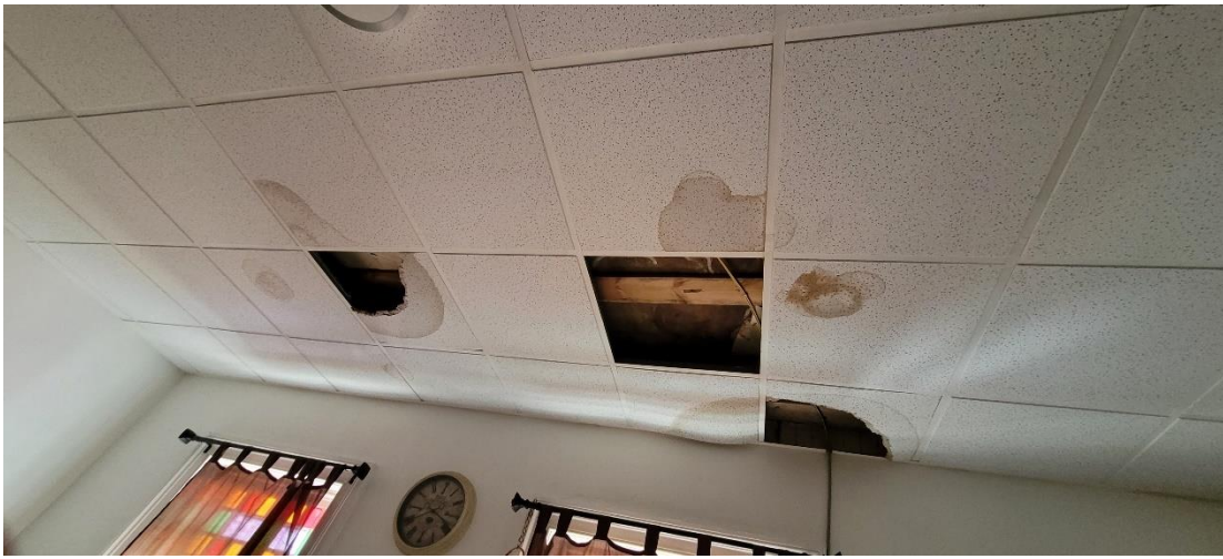
Figure 3: 36 King St. W – photo showing roof leak damage on the interior
