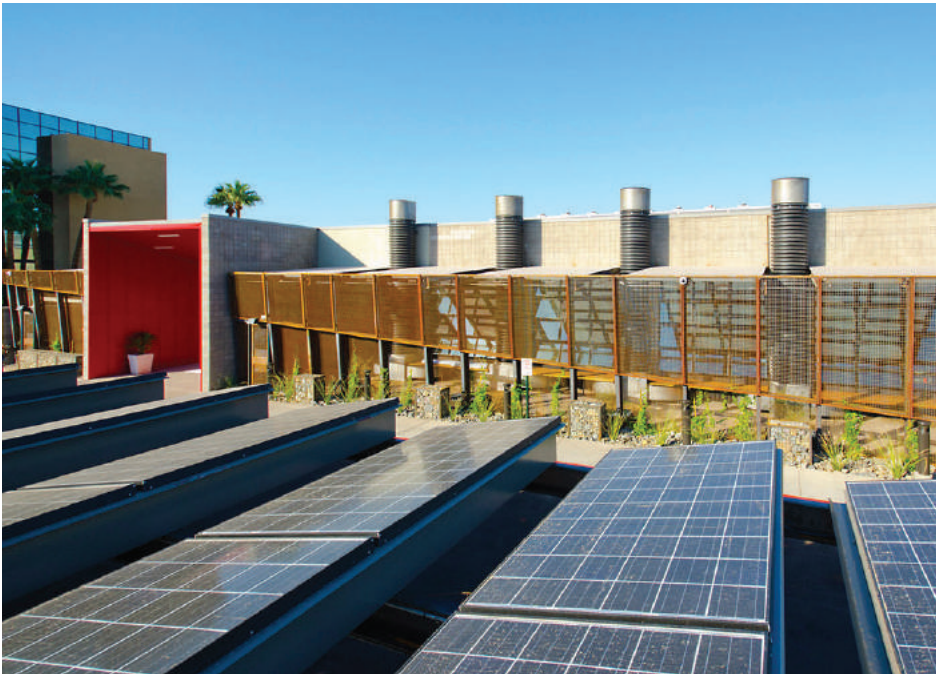
On-site energy production
