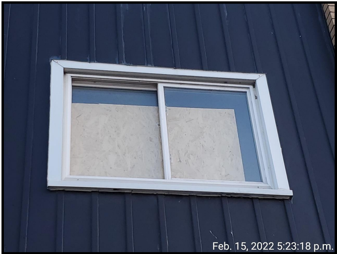
Figure 4: 9 King St. E infill building across the street with vinyl window. Photo provided by applicant.
