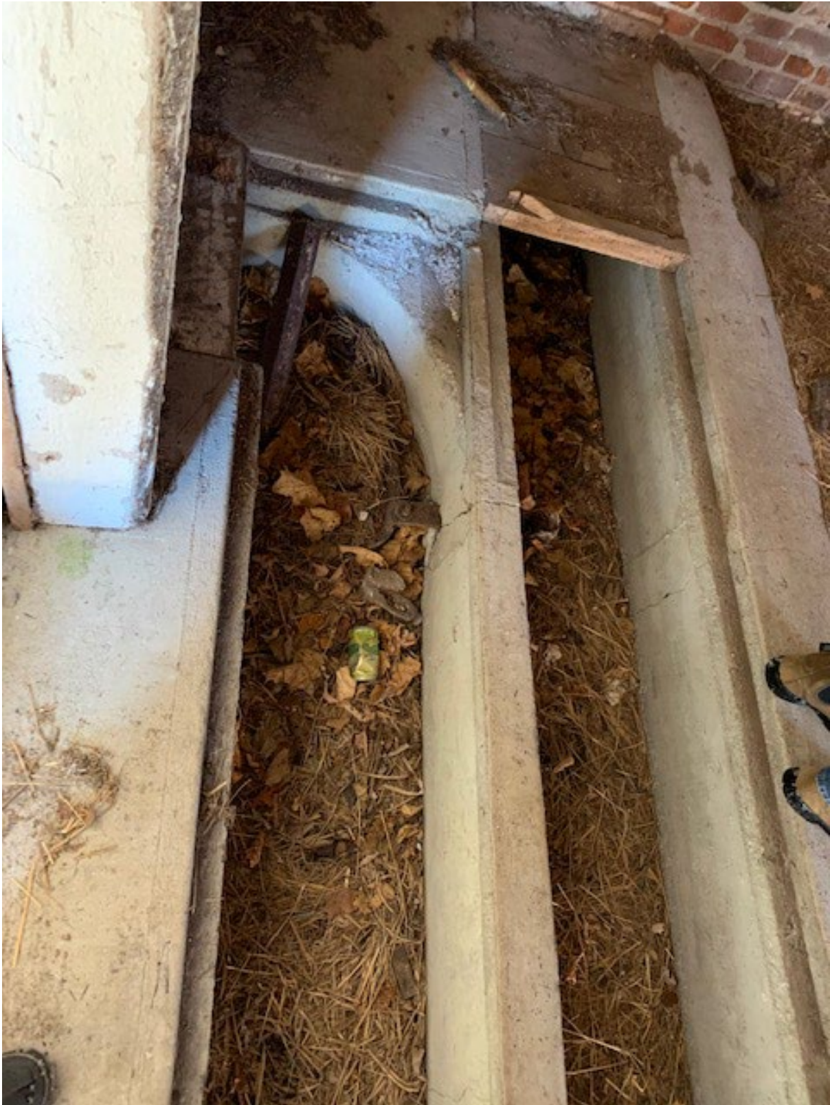
Double gutters in the byre for the “stable cleaner” manure-removal system
