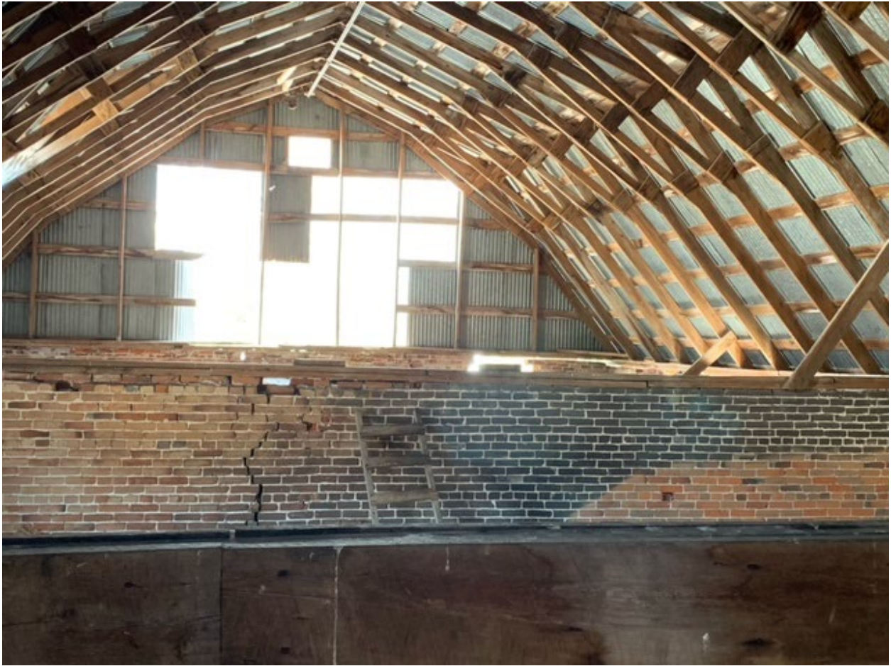
Looking east past the brick half-wall that may mark the east wall of the original barn, with the addition beyond
