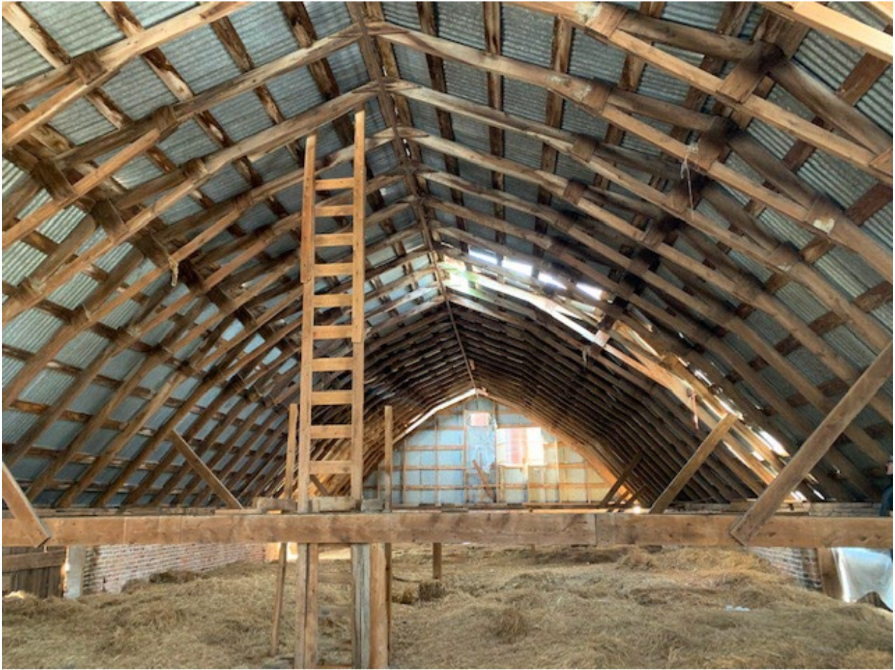
Looking toward the west end of the hay loft ("mow"), with silos beyond.
