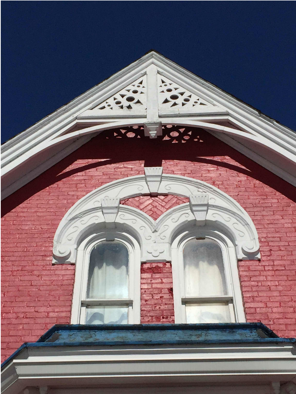
Paired round-headed windows over bay window with double hood-mould arches incorporating a herringbone brickwork inset, vergeboard fretwork and trusses in gable, and copper sheathing on roof of bay.
