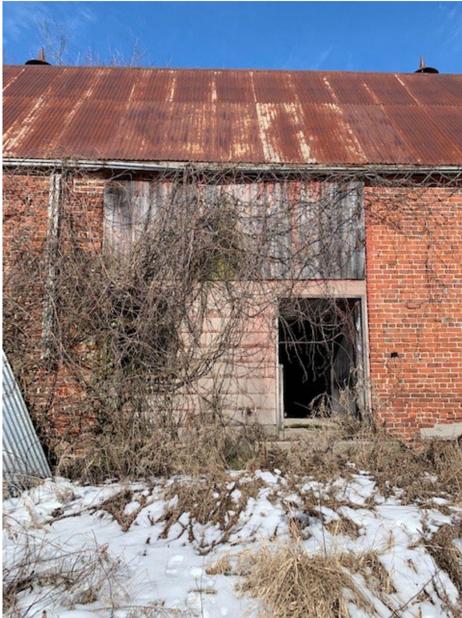
Location of the great cart doors in the centre section, south elevation.
