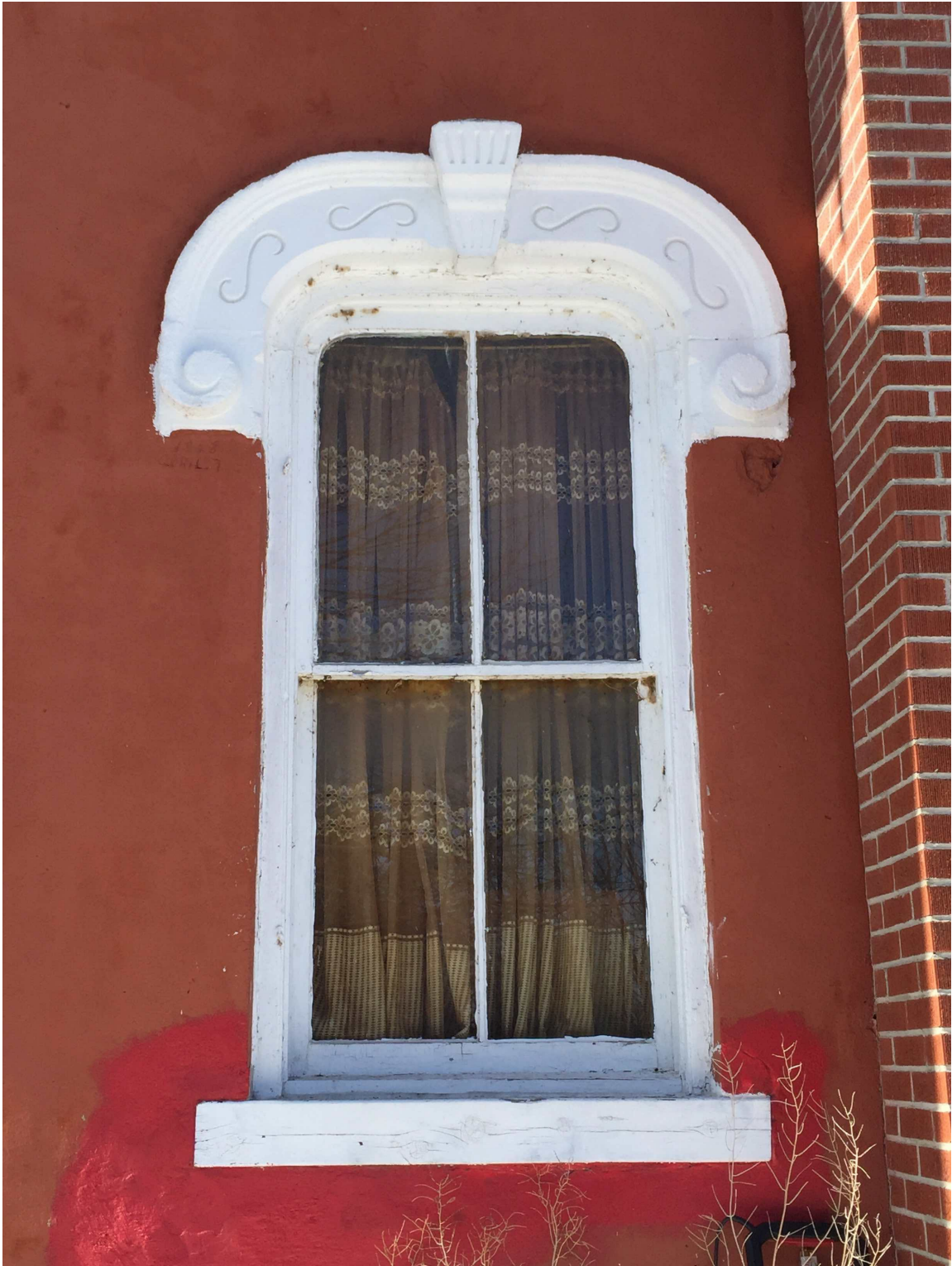
Ground-floor round-headed window with figured hood mould, keystone, and curlicues. East elevation. Note replacement chimney on right.
