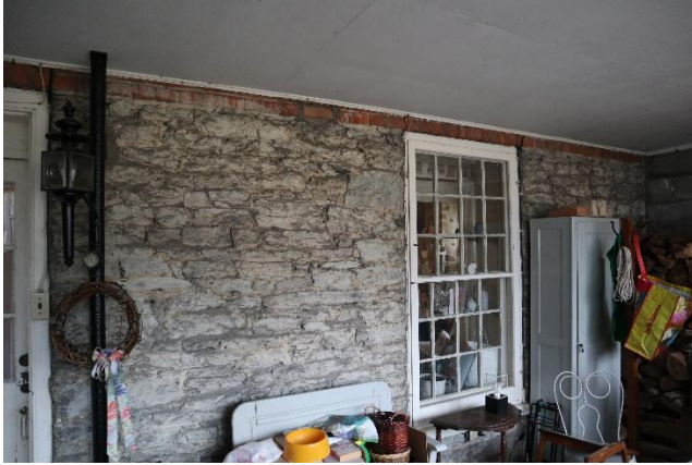
Figure 17. Photo of rear (south) elevation basement with the door seen on the left-hand side of the photo (photo taken by Planning staff during Feb 2024 site visit)
